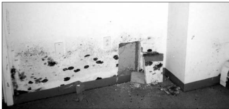
After the rain leakage test is performed on the building exterior, field engineers removed sections of the interior wall to see if water had leaked into the walls. Because it had not, we knew that condensation was the cause of the mold growth.
