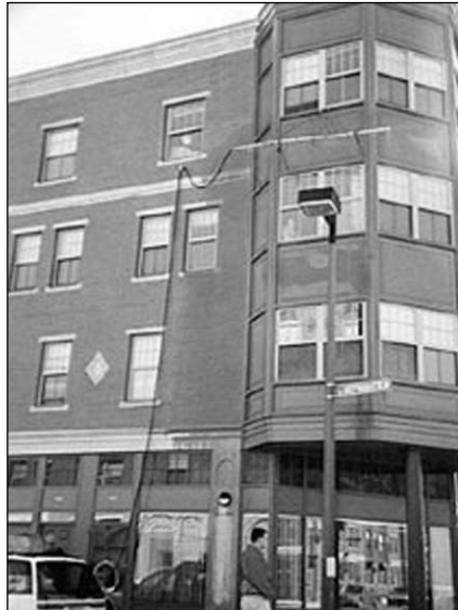
At Roxbury Corners, we performed a rain leakage test to determine if rainwater was leaking into the walls.
