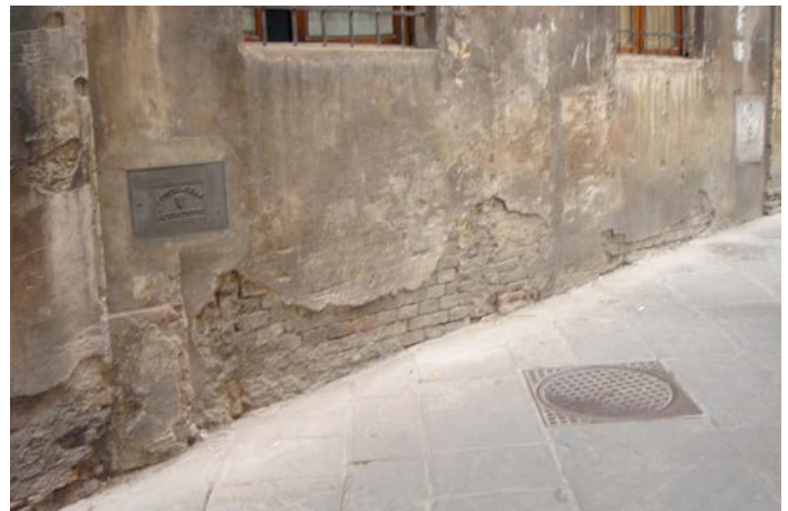
Photograph 2: Spalling of sacrificial layer in Siena, Italy
