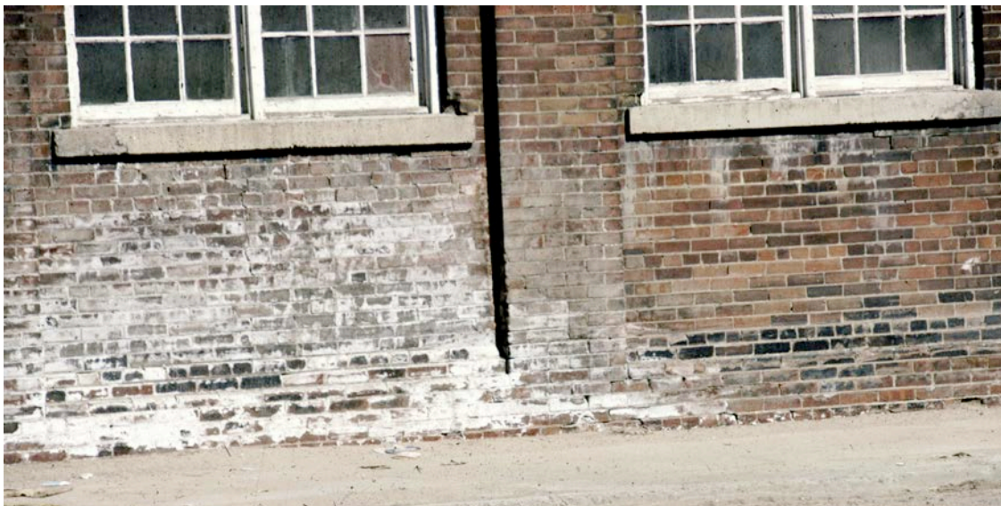
Photograph 1: Efflorescence on brick foundation
