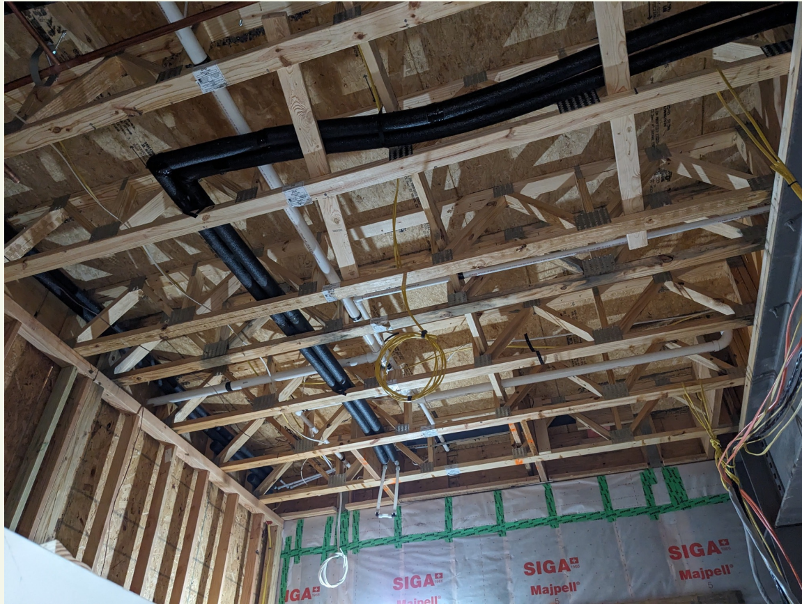
2-Pipe “line set” out to fan coil
