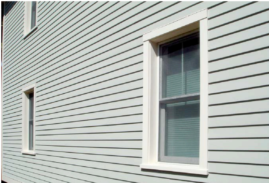
Photograph 1: Beautiful “Innies” — The trim is returned to the flange or face of the inset window. The flashing at the top of the window opening at the horizontal strip of head trim just covers the top of the trim itself—it only protects the top of the trim - it does not have to extend to the back of the continuous insulation and connect to the face of the structural sheathing/water control and air control layer.
