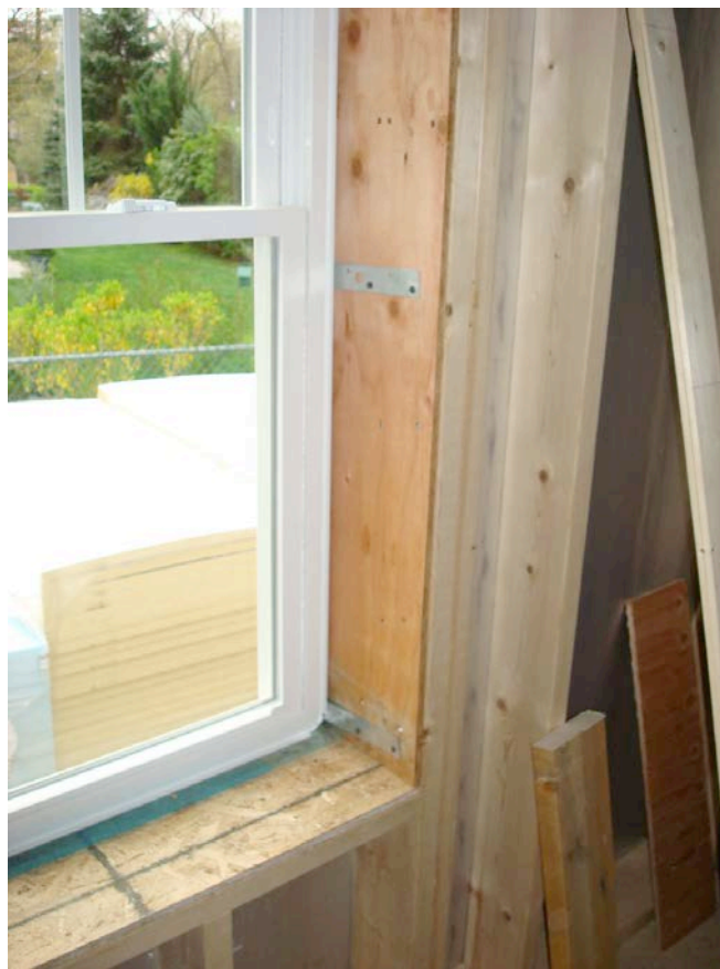
Photograph 3: Strap Window Attachment —Similar to window installation in masonry opens lined with window bucks. Unlike masonry openings the window flanges are retained for water control.
