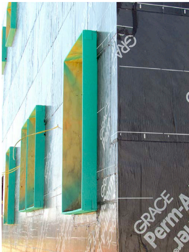
Photograph 2: Structural Box —Typically plywood or OSB protruding past the exterior face of the framing extending the thickness of the continuous insulation. How thick can you go with the continuous insulation with the structural box? Typically 4 to 6 inches.
