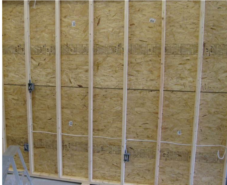
Figure 15 – Electrical Installed and Horizontal Gap Visible
