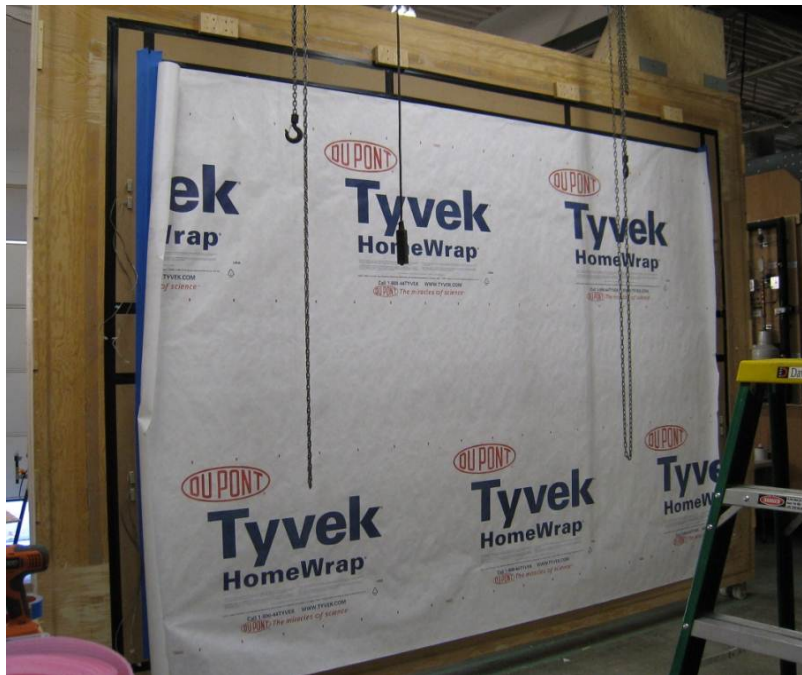
Figure 17 – Tyvek Installed but Untaped
