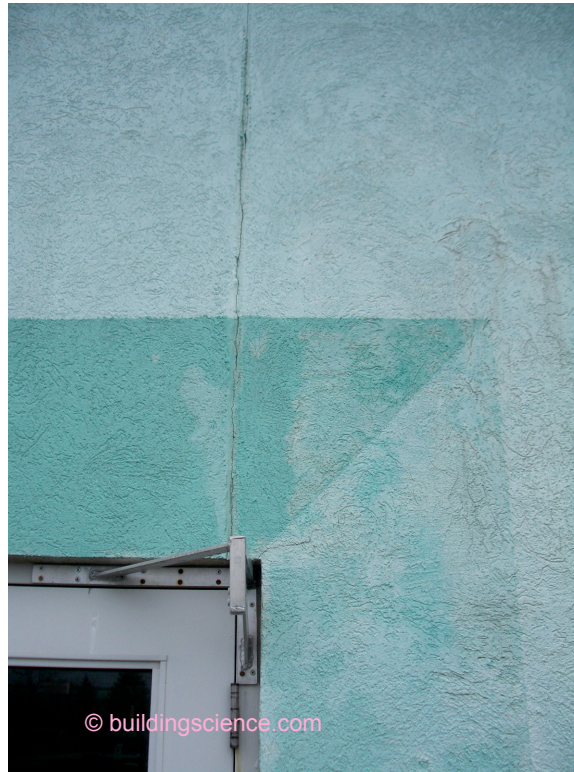
Photograph 2: Cracks in EIFS laminas are often found initially at reveals and at window openings
