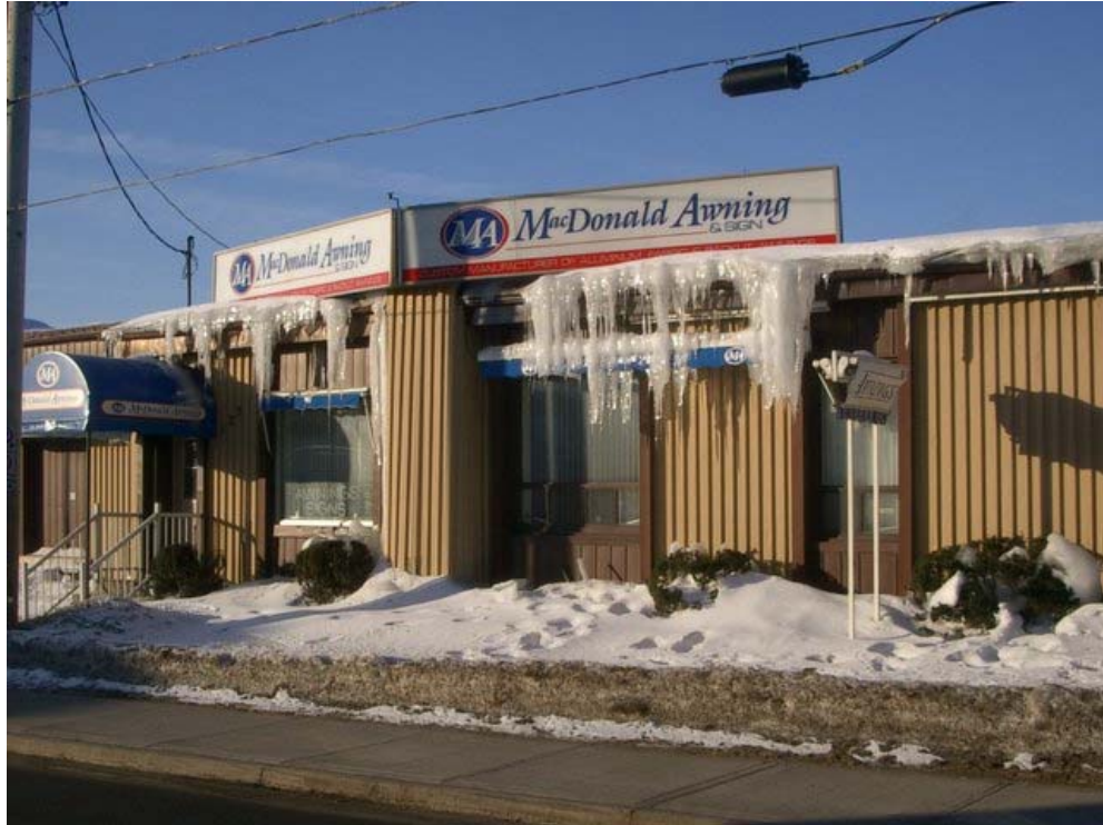
Photograph 2: Not just a problem for sloped roofs
