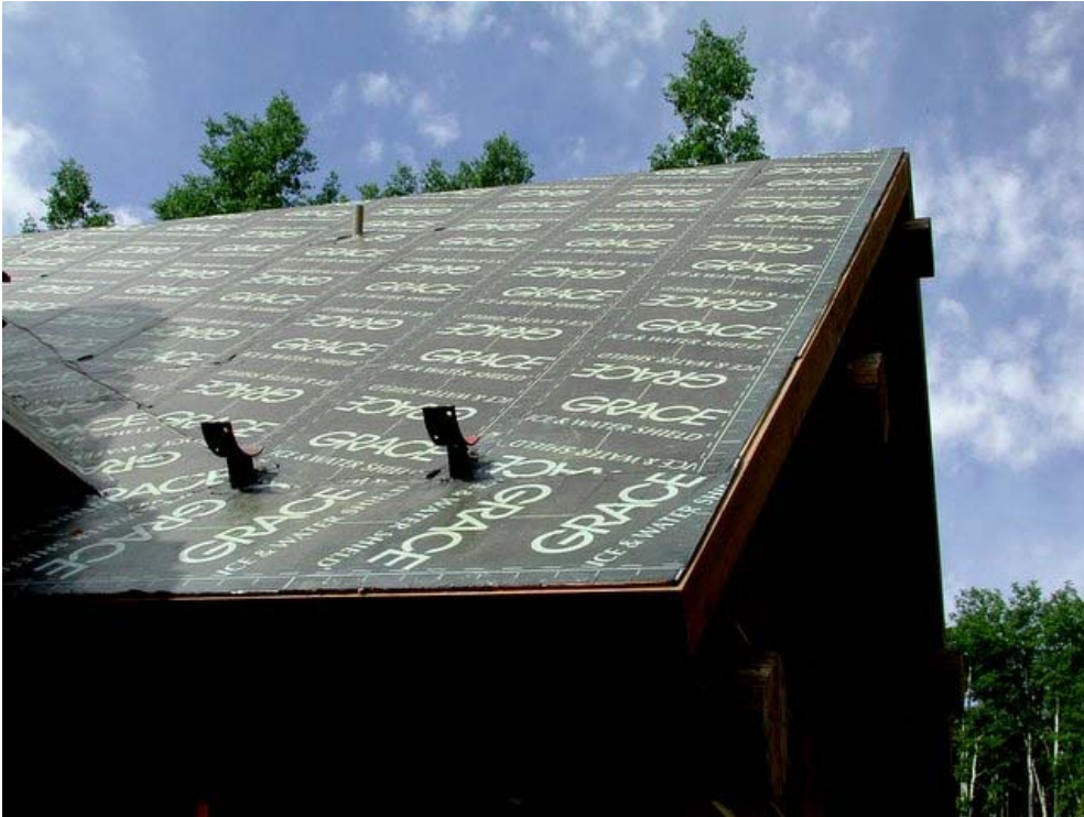
Photograph 6: Self-adhering membrane over the entire roof surface – an appropriate solution in some climates
