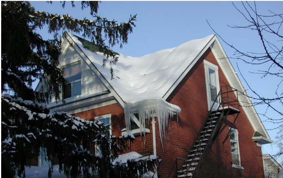
Photograph 1: An ice dam - note the snow melting on the slope above the ice dam.
