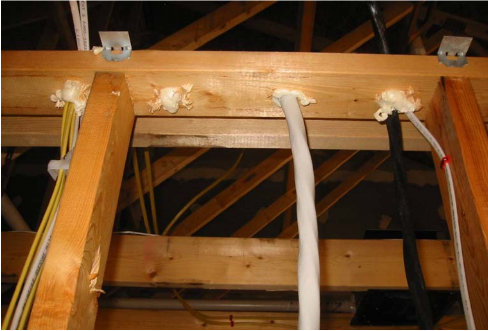
Photograph 5: Air-sealing with expanding polyurethane foam – much easier to do before the interior finishes are installed.
