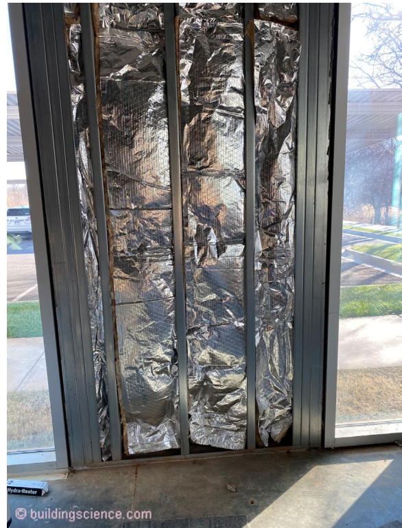
Photograph 7: Aluminum Foil on Cavity Insulation - aka “reflective insulation” on the inside of batt insulation? Nope, not a radiant barrier...a vapor barrier.
