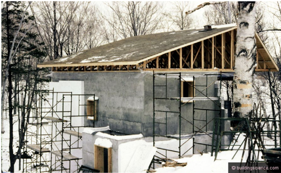
Photograph 1: Mass and Glass – A concrete block wall insulated on the exterior with 6 inches of expanded polystyrene. Note the “high heel” roof trusses so that ceiling insulation does not get “squeezed” at the perimeter. Yup, I did a few things correctly.
