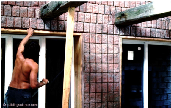
Photograph 2: Exposed and Coupled Interior Thermal Mass – Looks pretty good. Very expensive. Only the main floor thermal mass was coupled and distributed to the inside and solar gain. But, all the “light and tight” super insulated frame buildings I did later worked better and were much less expensive.
