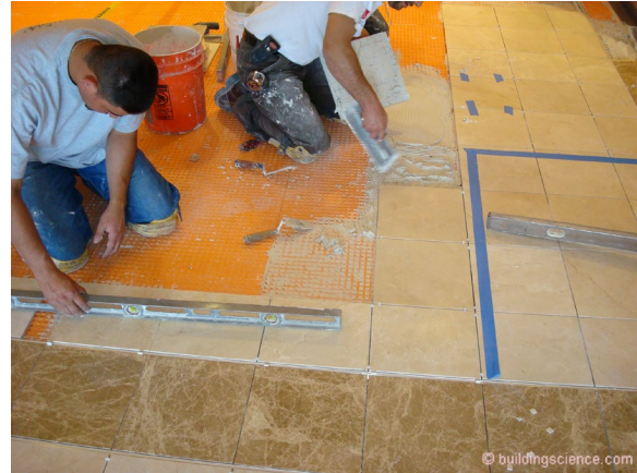
Photograph 9: Distributed Thermal Mass – Tile flooring...who knew...real impact on increasing the “time constant” of a “light and tight” well insulated frame house.
