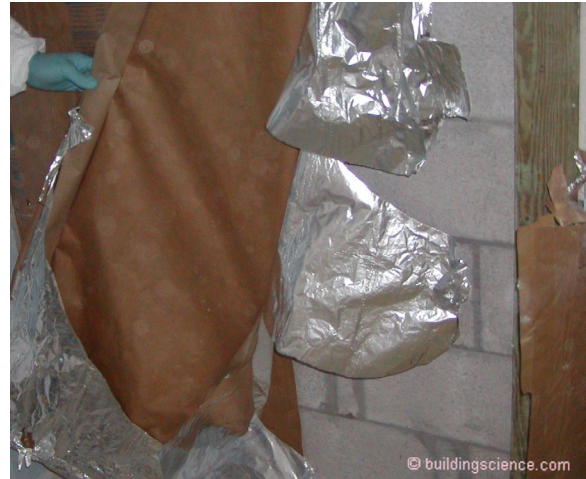
Photograph 8: Aluminum Foil on the Inside of a Block Wall in Florida – The “reflective insulation” was installed over \frac{3}{4} inch wood furring with the foil facing the airspace. The aluminum foil turned out to be a vapor barrier on the wrong side of the wall. Mold city.
