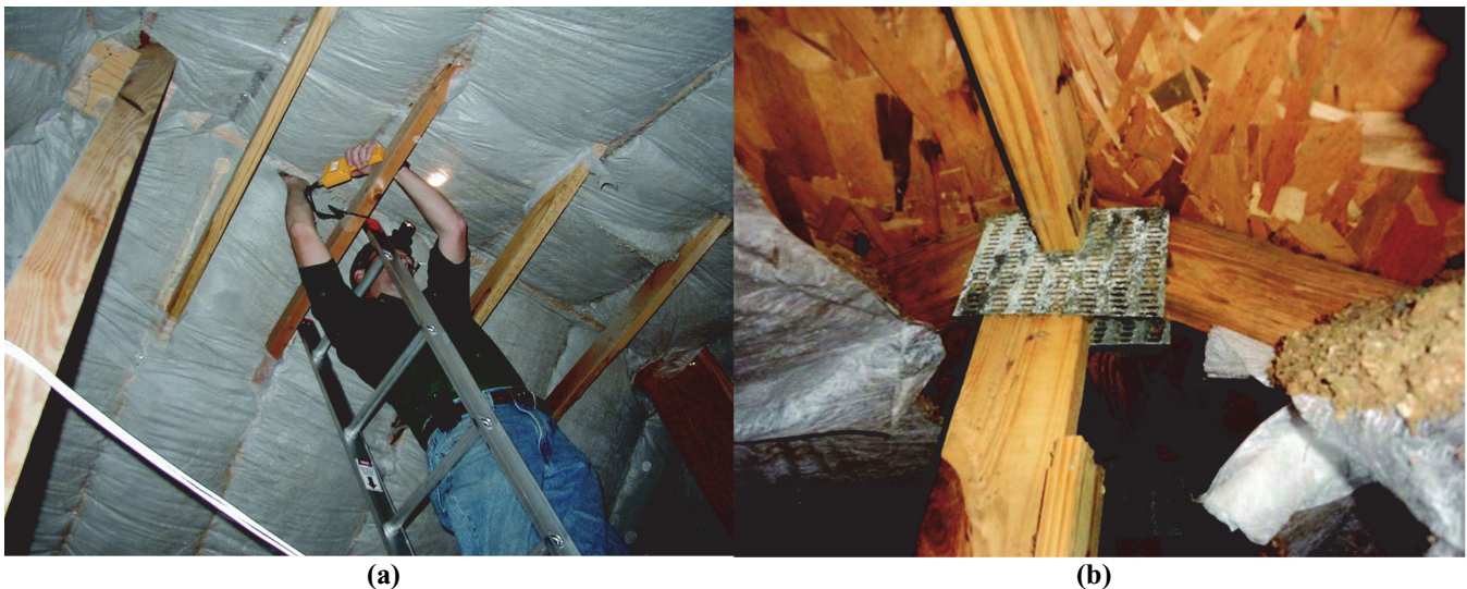
Figure 1 (a) Unvented cellulose roof ridge moisture content measurements in Houston, TX and (b) corrosion of ridge truss plate in Jacksonville, FL.
