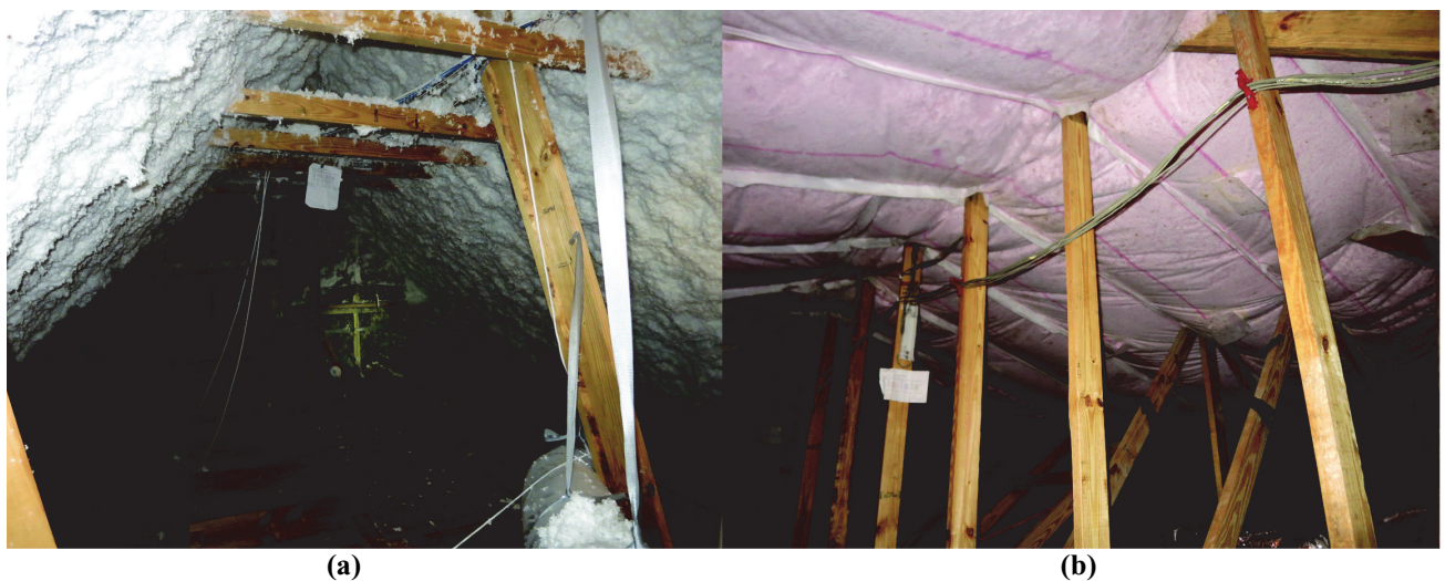
Figure 3 Attic interiors: (a) spray-applied fiberglass in Houston and (b) netted/blown fiberglass in Orlando.
