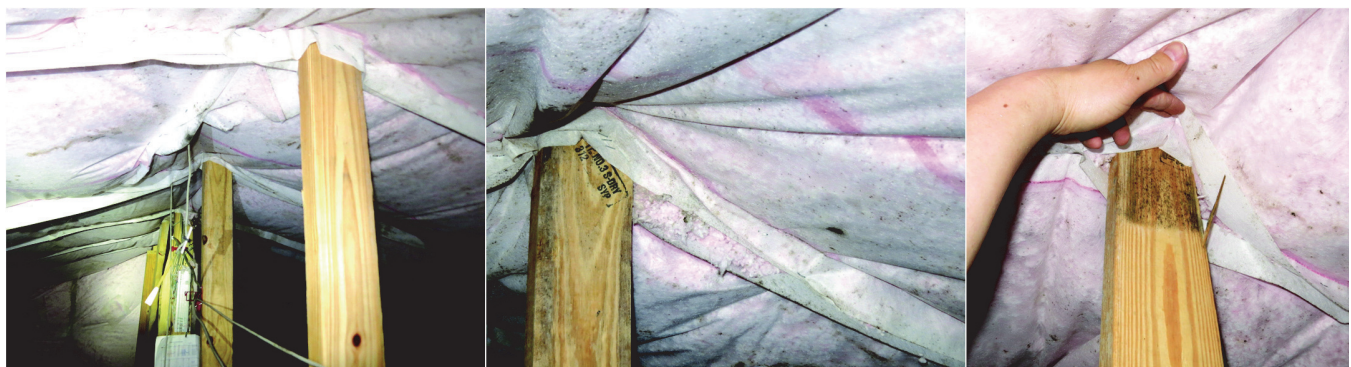
Figure 23 Orlando tile roof interior conditions showing spotting on insulation netting and truss vertical member.
