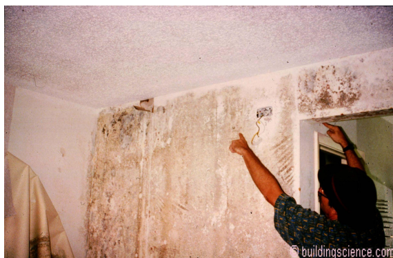
Photograph 9: Mold Damage on Interior Wall - The infiltration of hot humid air from the exterior through the hotel room demising wall ultimately ending up in the bathroom dropped ceiling leads to the mold damage shown.
