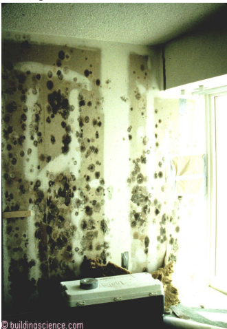
Photograph 6: Under the Vinyl Wall Covering – Hotel suite rooms were pressurized, demising walls were negative and coupled to the exterior air.
