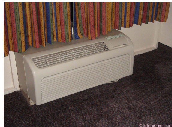
Photograph 2: “Through Wall A/C - Packaged terminal air conditioners “PTAC’s” or packaged terminal heat pumps “PTHP’s”.
