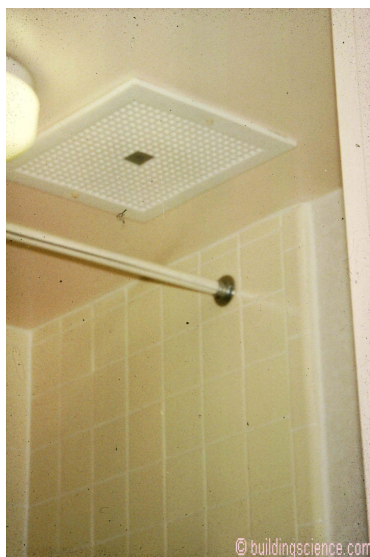
Photograph 7: Bathroom Exhaust - The exhaust grille unit is not airtight. The connection between the gypsum board and the edge of the exhaust grille unit is not airtight. The duct that extends to the shaft is not airtight. So the entire bathroom dropped ceiling area is negative.
