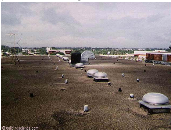
Photograph 1: Hotel Rooftop Exhaust - Air is extracted from each bathroom with rooftop exhaust fans. Each rooftop fan exhausts multiple hotel rooms. The rooms are typically “paired” to a neighboring room and the pairs “stacked” over each other with a vertical shaft connecting the bathrooms to the rooftop exhaust fan.
