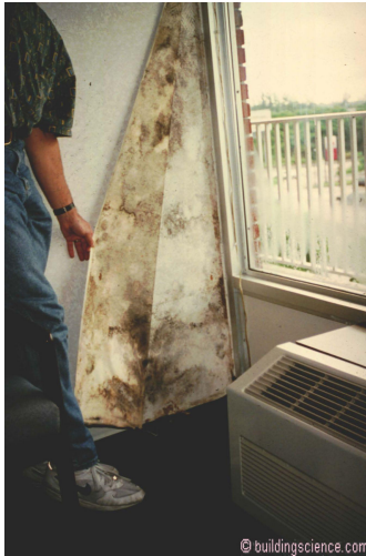
Photograph 5: More Vinyl Wall Covering – Again, this is on an interior demising wall.
