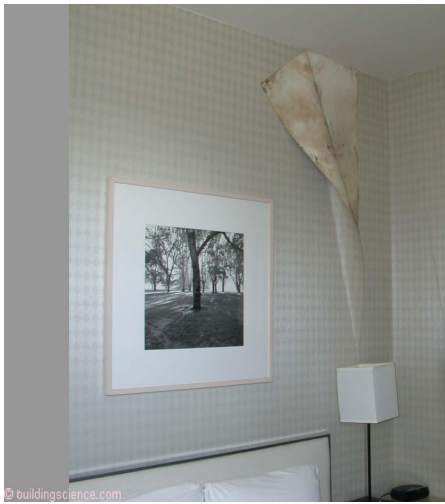
Photograph 4: Vinyl Wall Covering – The mold damage is on an interior demising wall.
