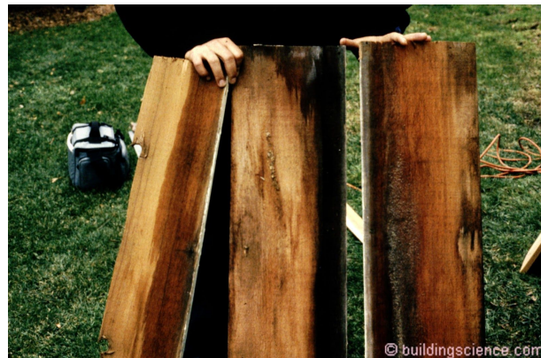
Photograph 3: Capillary Rise Between Lapped Wood Siding – Damage to wood siding from water trapped between the horizontal laps.
