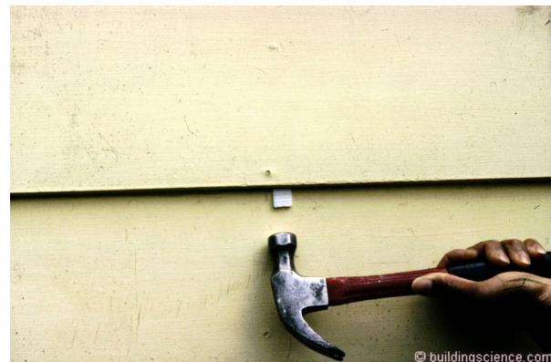
Photograph 6: Retrofit “Wedgie” - Siding can be gapped to provide a capillary break. Siding wedges have been used in the past to address peeling paint problems resulting from capillary rise between overlapping siding.
