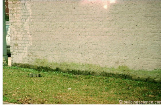
Photograph 1: Capillary Rise in Pores - Ground water is drawn into porous brick in contact with the ground. Mother Nature, in her effort to educate builders and architects, thoughtfully provides chlorophyll as a tracer pigment in this case to illustrate capillary rise.
