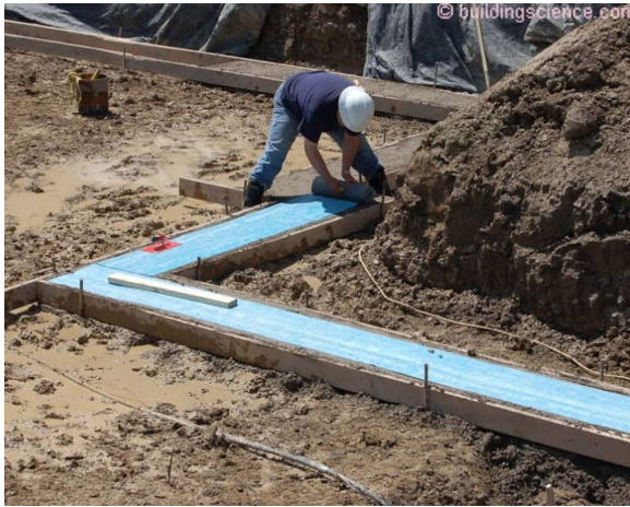
Photograph 5: Footing Capillary Break – Membrane applied capillary break located over the top of concrete footings prior to the construction of perimeter foundation walls.
