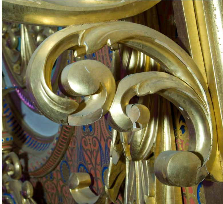
Smaller gilding defects
