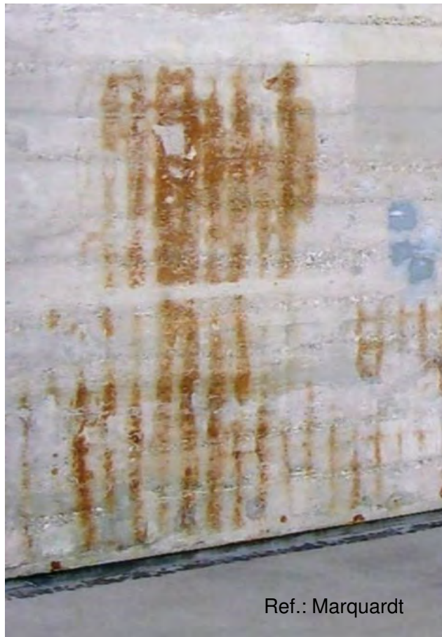
Corrosion of concrete sandwich element after carbonation of exterior surface layer
