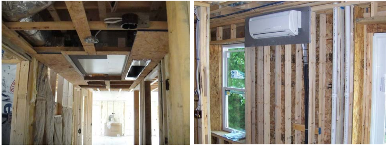
Figure 2 Minimally-ducted mini split mounted in dropped ceiling space (left) and single-point wall-mounted ductless split indoor unit (right)
