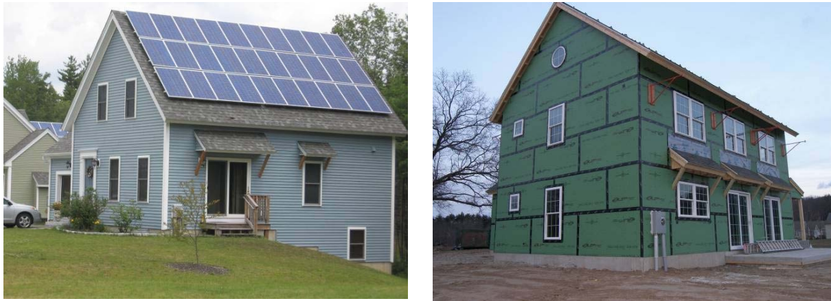
Figure 1 Completed house example (left), and house under construction, showing exterior air barrier approach (adhesive tape sealed seams on exterior sheathing) (right)
