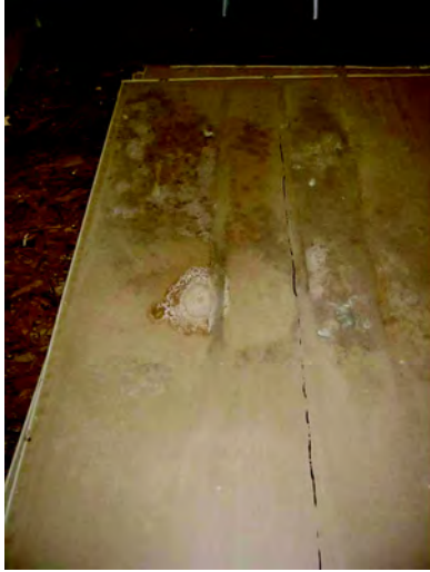
Figure 17 Mold on brick west wall gypsum wallboard.
