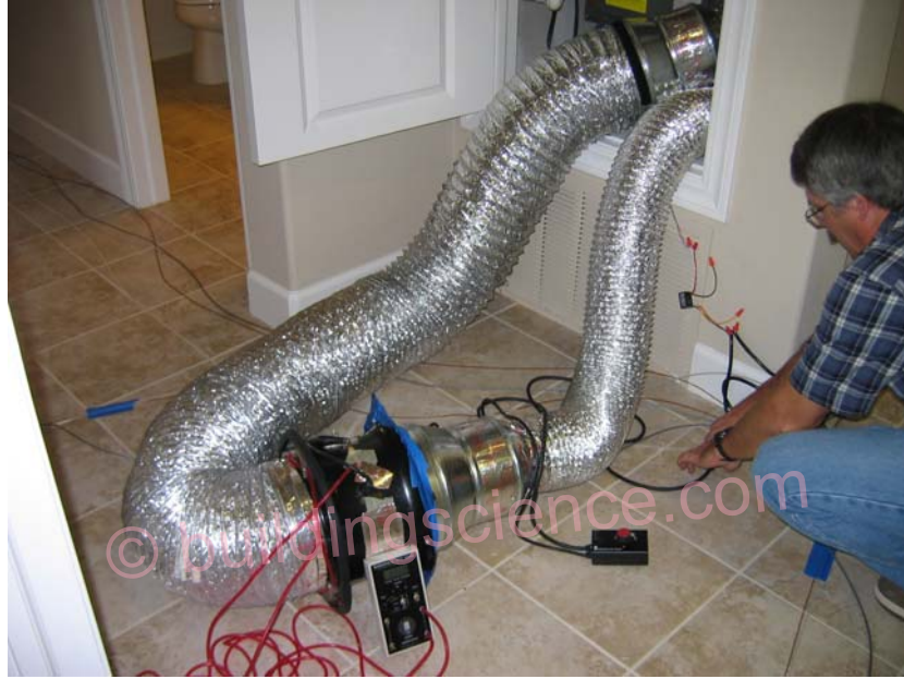
Figure 8. Duct Blaster installed between the outside air duct and the return of the air handler to provide supply ventilation.
