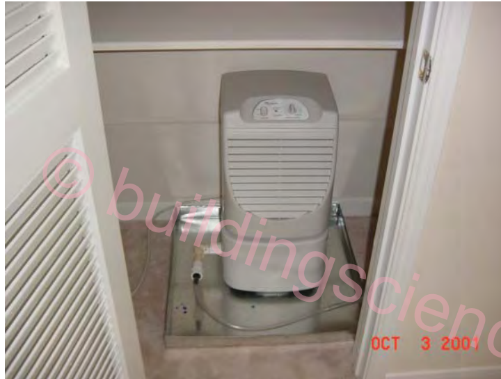
Figure A-1a. Photograph of stand-alone dehumidifier in hall closet with louvered door system
