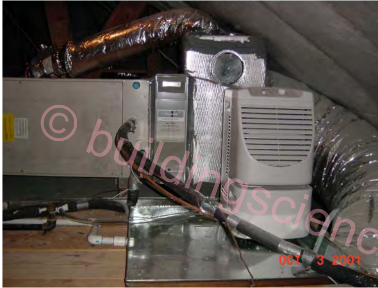
Figure A-2a. Stand-alone dehumidifier in conditioned attic
