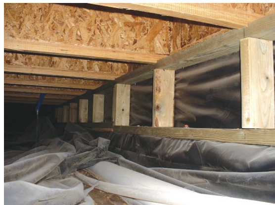
Figure SC-7: Conditioned crawlspace
