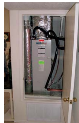
Air handler closet located in hallway
