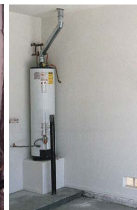
Garage installation of water heater
