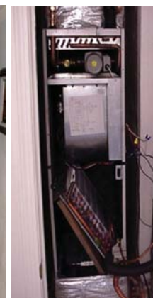
“Guts” of the air handler with heat exchanger
