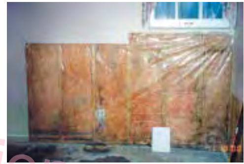
Photograph 5 Frame wall with interior vapor barrier resulting in mold, decay and odors
