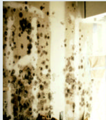
Mold growth on vinyl wall covering.
