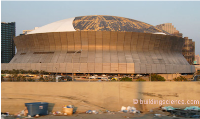
Photograph above: Should Have Never Happened-The Superdome roof membrane is missing after Hurricane Katrina.
