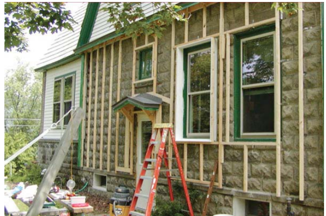
Photograph 13: Wood Frame Off-Set Residential Retrofit —Pretty neat, eh? My friend Peter Yost’s house in Vermont prior to installation of SPF.
