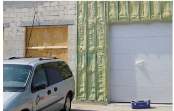
Photograph 10: Light Industrial Strip Mall —Masonry wall insulated on the exterior with spray foam. Note the treated wood 2x2 furring on screw offsets.
