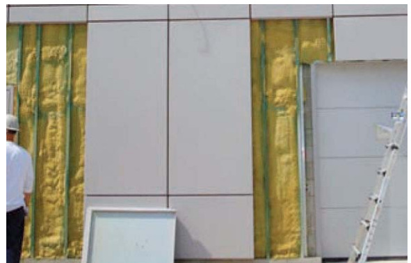
Photograph 11: Steel Panel Cladding —Steel panels installed onto wood 2x2 wood furring embedded in spray foam on masonry wall enclosure for a light-industrial strip mall.
