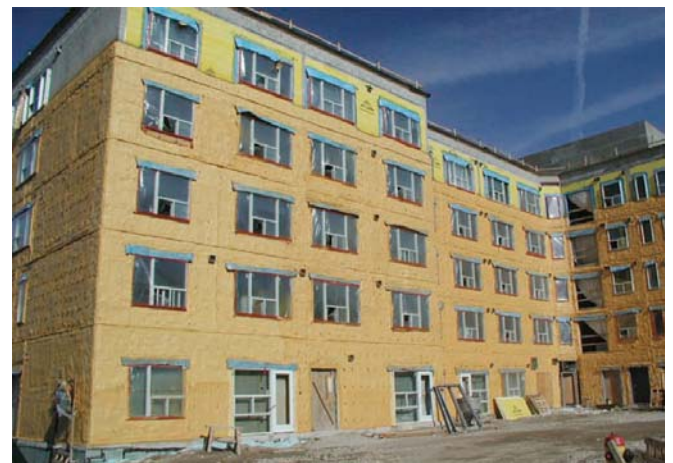
Photograph 1: The Perfect Wall?
