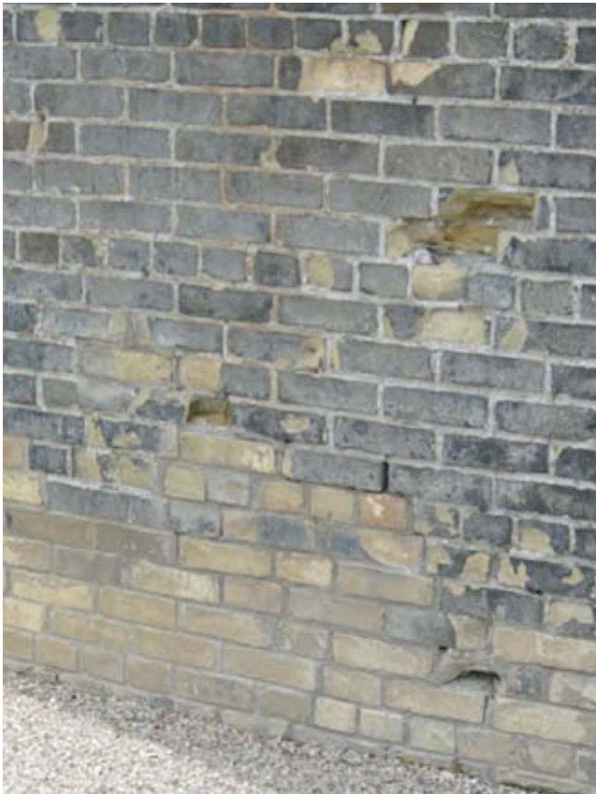
Photograph 2: “Classic” Freeze/Thaw Damage —Low to the ground, not very exposed to rainwater and in really bad shape. It turns out that this is a “bad” brick with a low S_{crit} .
