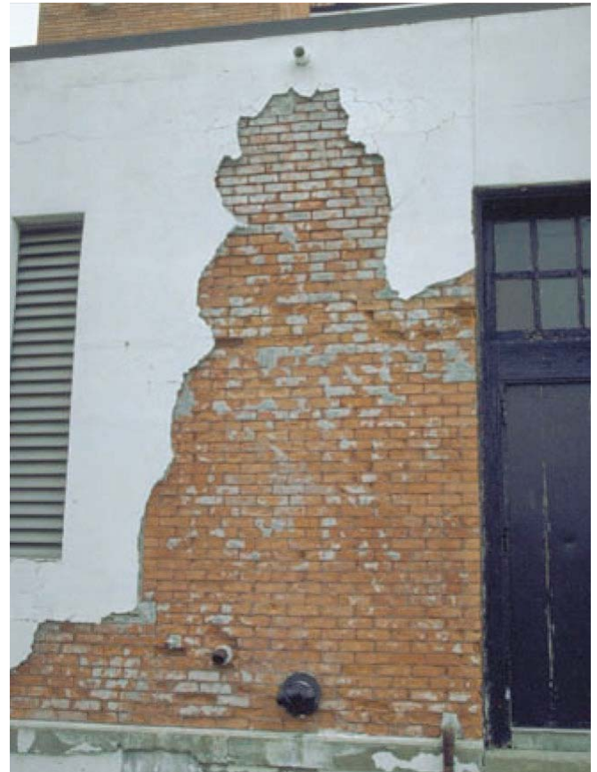
Photograph 3: Scupper —This is a no brainer. Don’t dump the roof water onto the wall. This is not an insulation problem. This is just dumb.
