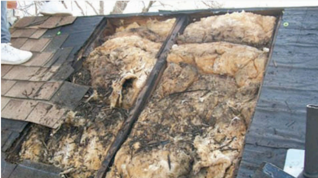
Photograph 6: Unvented Cathedral Ceiling —No one argues that it is a dumb idea to shove a bunch of fiberglass batts into a cathedral ceiling with no provision for ventilation air to remove some moisture. The results are often catastrophic.
