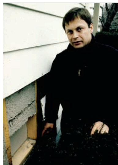
Photograph 5: Real World Wall —A young engineer in Cleveland 25 years ago who didn't believe that you could retrofit blown insulation into a wall cavity and make it work. I opened up more wall cavities than I would like to admit. Two things happened. I became a believer in dense packing walls, and, wait for it, I became a fan of Cleveland. Who knew? Shame on you, LeBron.
