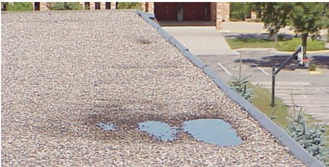
Photograph 7: Flat Roof —There are a gazillion of these roofs that are uninsulated and need to be addressed.
