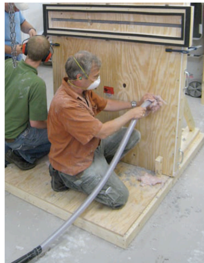
Photograph 2: Skunk Works Air Leakage Testing —They only work this hard when we have a camera and the boss is around. A test wall cavity is being insulated with “dense pack” insulation.
