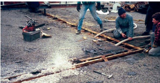
Photograph 8: Flat Roof Being Dense Packed —The roof is opened up and cellulose is being blown into the roof cavity dense packing it. The guy in the middle is Jim Fitzgerald, the absolute best guy in the world, and he could not make it work consistently. Does that tell you something, or what?
