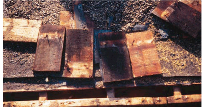
Photograph 9: Damaged Decking —The proof of the insulating is in the opening (old insulation contractor proverb). The deck did not stand a chance. Don't do this.
