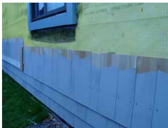
Photograph 4: Cedar Shingles —Back ventilation and drainage of wood shingle cladding installed over OSB covered housewrap – it does not get better than this from a durability perspective.
