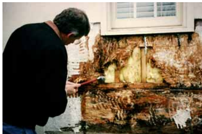
Photograph 8: Nightmare —Exterior Insulated Finish System (EIFS) directly adhered to water sensitive OSB sheathing. Water passes through and around stucco cladding and is trapped between the foam sheathing and the OSB. Water-managed EIFS does not have this problem and is an awesome system.
