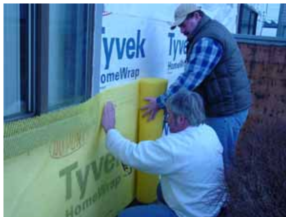
Photograph 3: “High-tech air?” —Polypropylene mesh providing an air gap between OSB covered with housewrap and cladding.
