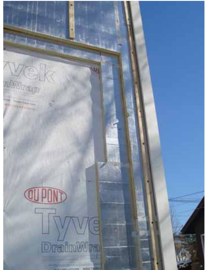
Photograph 11: Perfect Wall Redux —The almost perfect wall has “crinkled” housewrap providing hygric redistribution, 4 inches of foil-faced polyisocyanurate insulating sheathing providing the ultimate thermal break, wood furring providing cladding attachment, relief of hydrostatic pressure and back-ventilation of cladding. OSB under the housewrap provides shear and high-density spray foam cavity insulation (obviously hidden from view) provides air sealing and even more thermal performance. Who says that all these products can’t get along?
