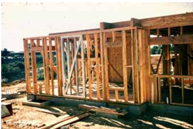
Photograph 6: Shear Resistance —Pre-manufactured metal inset shear panels are quite common in high seismic risk zones.
