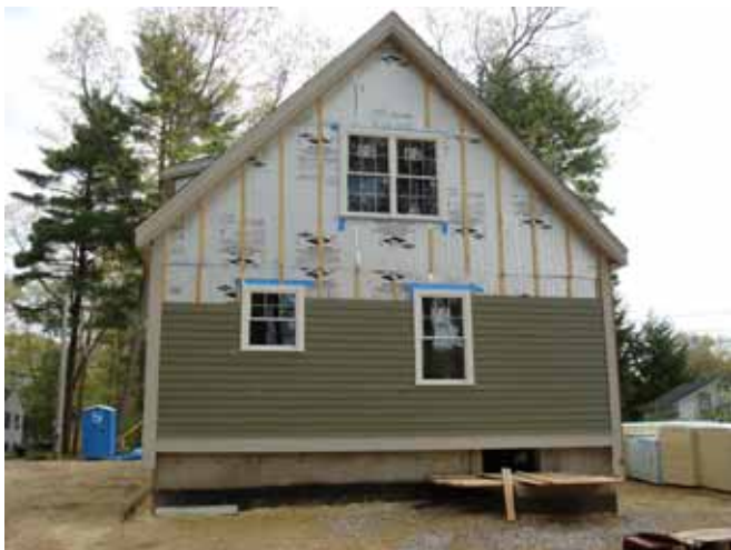
Photograph 7: Furring —When foam sheathings exceed 2 inches in thickness 1x4 furring becomes necessary. This wall has 4 inches of foil-faced polyisocyanurate insulating sheathing installed over a 2x6 wood frame wall. The wood furring acts as the nail base for the fiber-cement cladding.
