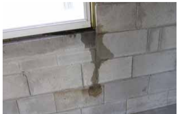
Photograph 4: Leakage Path —Yes, they all really do leak; at the window-to-wall interface and through the window itself.
