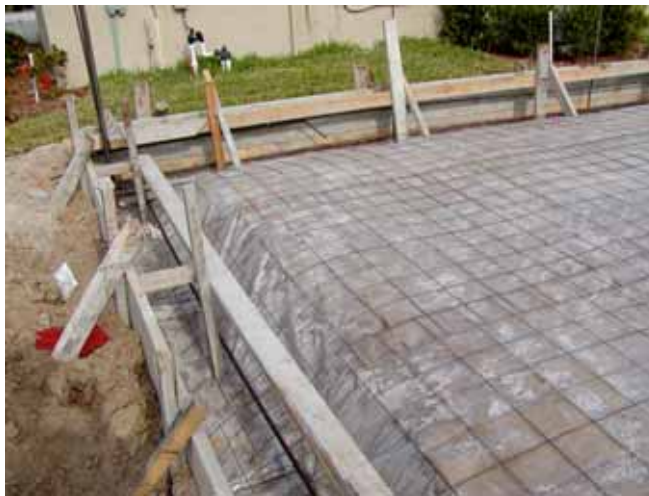
Photograph 2: Perimeter Capillary Break —Plastic sheet extends out under perimeter of slab edge foundation. Plastic skirt is attached to perimeter form boards protecting below grade portion of exterior slab edge.
