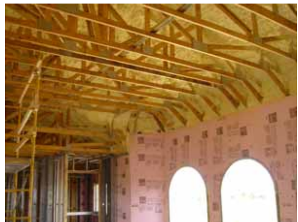
Photograph 5: Unvented Roof —Spray foam insulation applied to the underside of the roof deck bringing the attic and the ductwork inside the conditioned space.
