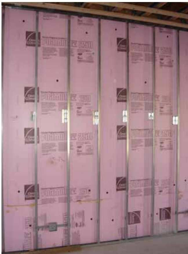
Photograph 3: Vapor Semi-Permeable Rigid Insulation —Note the steel stud interior wall framing is supported by brackets that do not penetrate the foam insulation but are installed over the top of the foam insulation.
