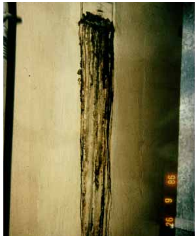
Photograph 5: Condensate Exiting Chimney Clean Out – Big danger here. Old oil furnace is replaced with a new gas furnace. New gas furnace uses existing chimney. Existing chimney is too big. Flue gases cool too quickly leading to condensation of flue gases and freeze up. How to fix this problem? Line the chimney – See Photograph 8.
