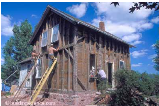
Photograph 2: Exposed Timber Frame —One hundred and fifty year timber frame house being renovated. Exterior horizontal sheathing boards and weatherboards removed. Note the close spacing of the vertical intermediate posts.
