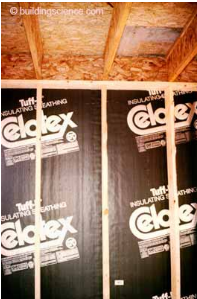
Photograph 5: Building America —Advanced frame 2x6 structure, studs on 24 inch centers, single top and bottom plates, 1.5 inches foil faced polyisocyanurate insulating sheathing. Cavity insulation not yet installed. This is likely to be the industry standard in the next decade. R&D courtesy of the US DOE Building America Program.
