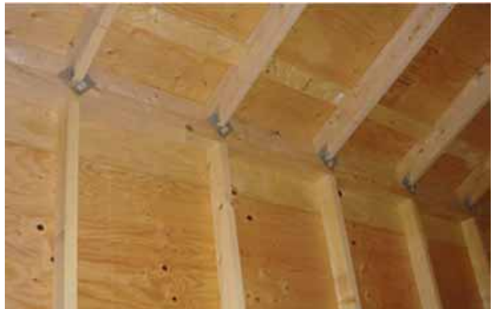
Photograph 5: Interior Structural Frame —The wood-frame wall cavities and wood rafter roof cavities remain uninsulated to control cavity condensation. The cavities provide space for services. The air barrier membrane and vapor barrier membrane are exterior to the wall and roof framing.
