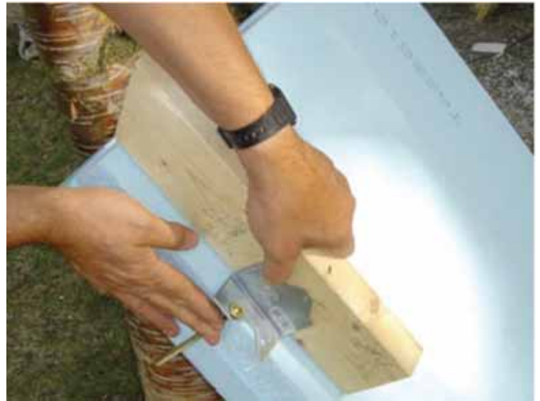
Photo 3: Ventilation Rafter —The 2x4 (standing proud) is connected through the roof rigid insulation with a metal bracket and a long roofing screw. You can purchase 14 in. (356 mm) long epoxy-coated steel screws. Stay away from stainless steel screws because the heads twist off. Stainless steel tends to be soft. Ask me how I know.
