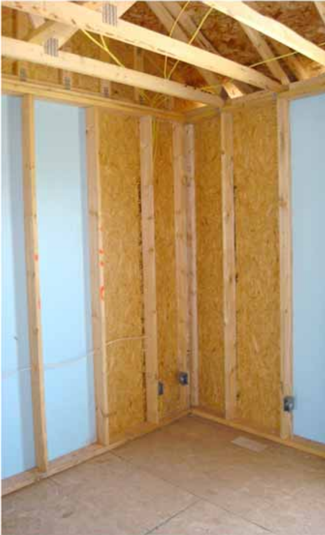
Photograph 7: OSB Braced Wall Panels - Insulating sheathing provides no “racking resistance” or “shear” properties. For that we need OSB or plywood braced wall panels – and most builders build them into corners.
