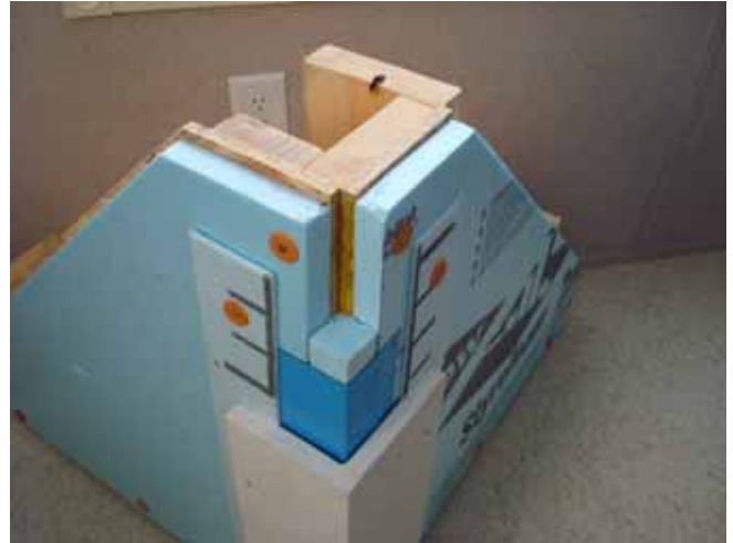
Photograph 8: Corner Framing With OSB and Insulating Sheathing – Note that the foam sheathing is reduced over the OSB shear panel so that the thickness of both sheathing layers line up with the thickness of the sheathing in the field of the wall. Also, note the spacer strip between the cladding and the exterior face of the insulating sheathing to provide back ventilation and drainage of the cladding layer and trim.
