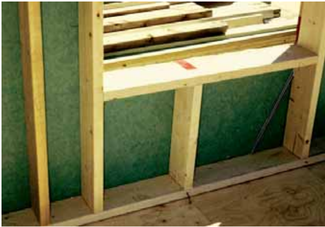
Photograph 2: Window Opening - Non-load bearing wall window openings are clean without jack studs and cripples.
