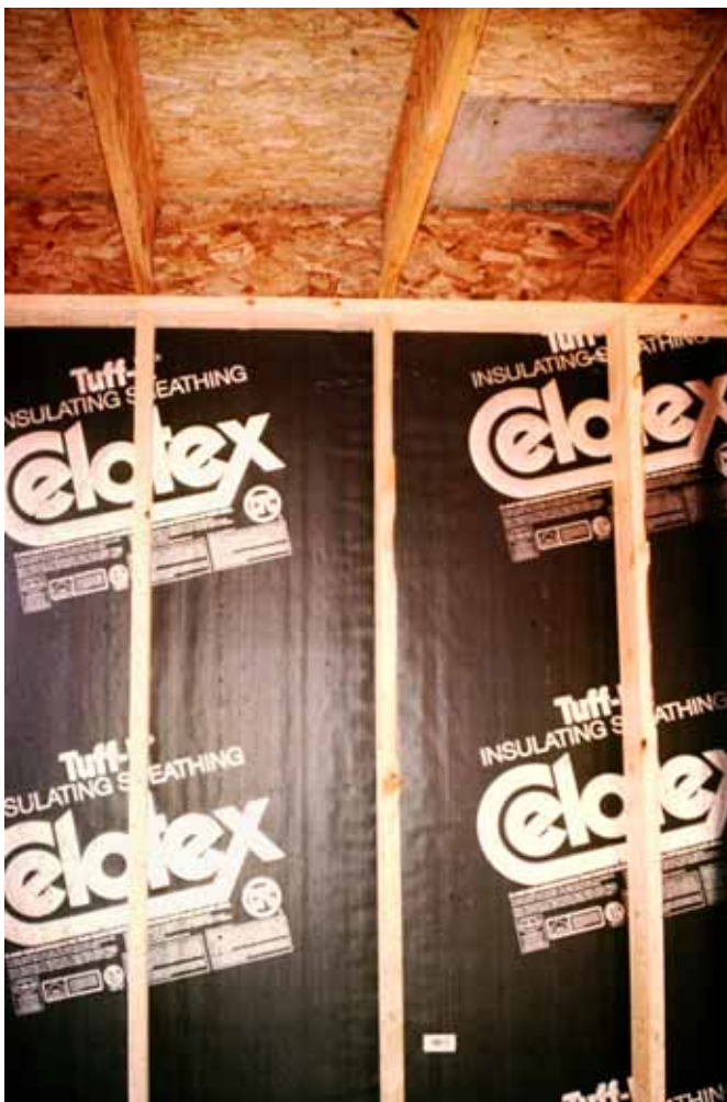
Photograph 1: Stack Framing - Everything lines up so that double top plates are not necessary.
