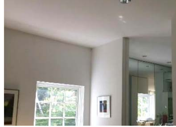
Vented attic above
