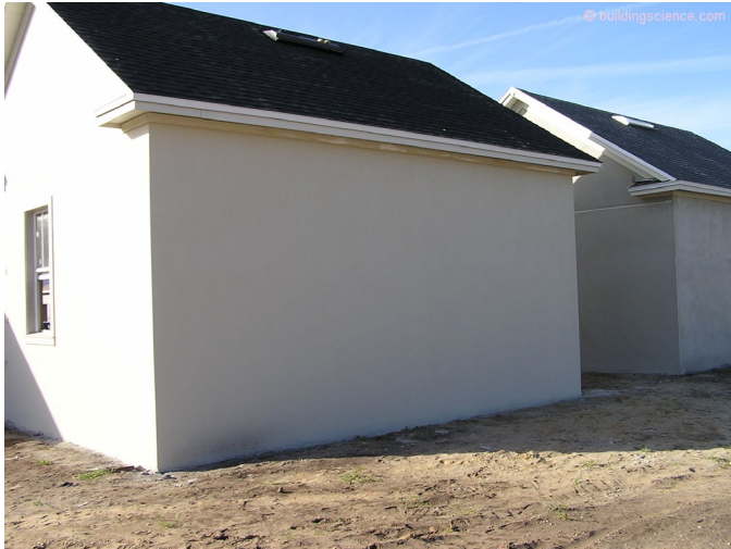
Photograph 1: Detached Garages - Playing with a row of detached garages with stucco over block construction.
