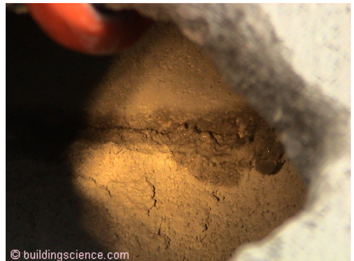
Photograph 4: Water Leakage - The suckers leaked after a couple of minutes – right into the block cavities. Not a couple of hours. A couple of minutes. Ten to fifteen minutes.
