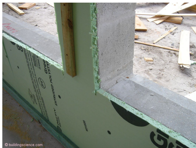
Photograph 7: Rigid Insulation Vapor Throttle - It is fairly common to use extruded polystyrene (XPS) rigid insulation on the interior of stucco clad CMU “block walls”.
