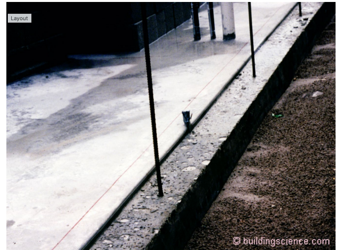
Photograph 8: Base of Wall Flashing – Installing a “seat” in concrete slab at the perimeter handles the rainwater draining down the CMU block cores. The “seat” acts as flashing directing the rainwater to the exterior of the wall.
