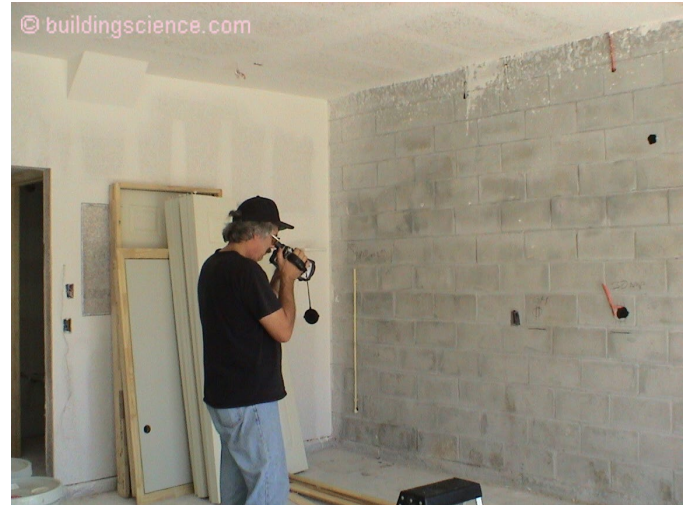
Photograph 3: Endoscopy for Walls - Knocked a bunch of holes on the inside of the block walls and looked inside.
