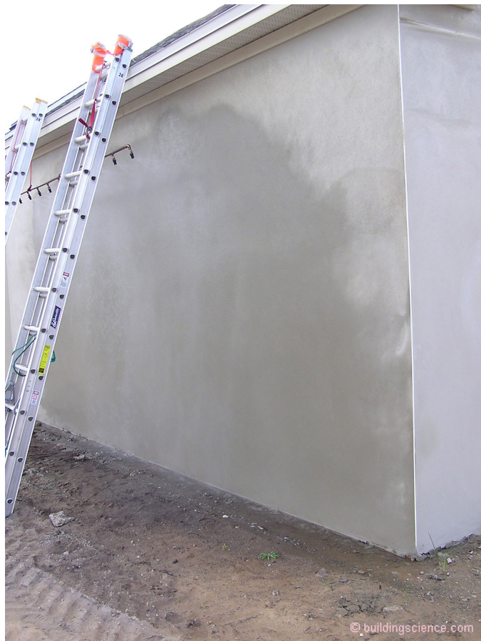
Photograph 2: Spray Rack – Adding water to the stucco surfaces at the ASTM E1105 5 gph/ft2 rate. No induced air pressure, just gravity, surface tension and capillarity.
