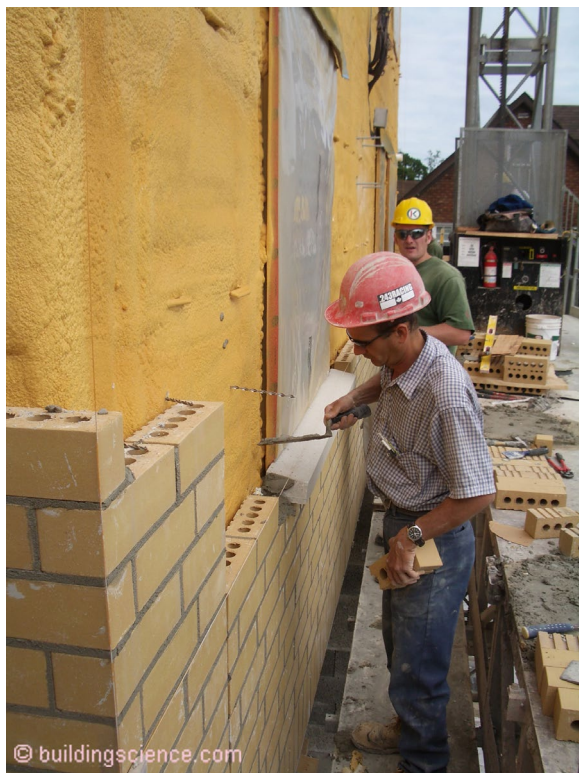
Photograph 6: Spray Polyurethane Foam - When you spray closed cell, high density spray polyurethane foam (ccSPF) on the exterior of gypsum sheathing or plywood or OSB it can act as the water control layer, air control layer, vapor control layer and thermal control layer....all four control layers
