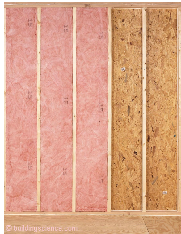
Photograph 10: Fiberglass and Mineral Wool Batts – When they are installed in wall cavities, roof cavities, on the ceilings of attics or on the underside of roof/attic sheathing they can’t act as the water control layer, the air control layer or the vapor control layer. They can act as the thermal control layer if airflow through them is limited or controlled.
