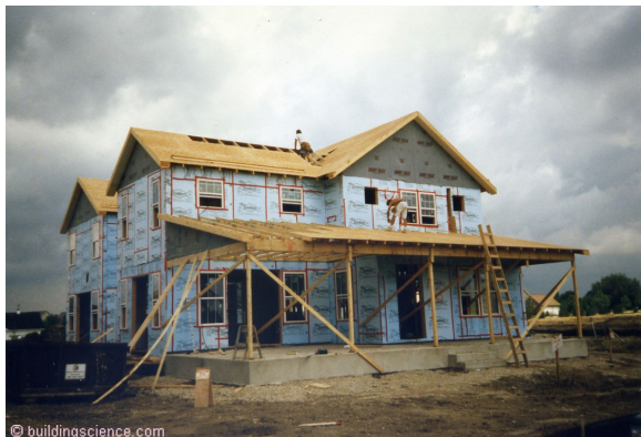
Photograph 2: Extruded Polystyrene (XPS) Boards - The rigid insulation boards are installed on the exterior of framing with their joints taped/sealed
