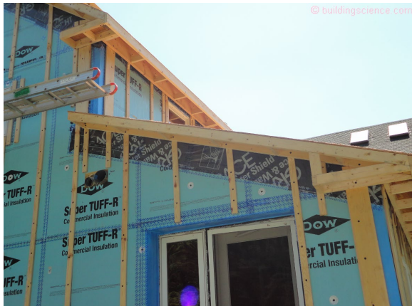
Photograph 1: Foil Faced Polyisocyanurate Boards – The rigid insulation boards are installed on the exterior of framing with their joints taped/sealed and act as the water control layer, air control layer, vapor control layer and thermal control layer....all four control layers.
