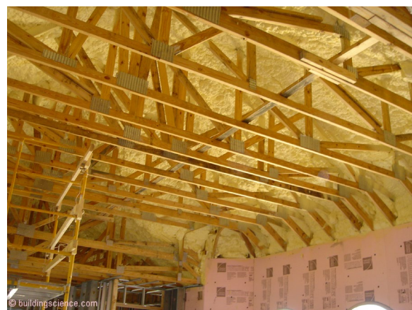
Photograph 8: Open Cell Spray Polyurethane Foam (ocSFP) - When you spray ocSPF into wall cavities from the interior the ocSPF can act as the air control layer and thermal control layer. It can't act as the vapor control layer - it is too vapor open. This is a problem when you spray ocSPF on the underside of roof/attic assemblies you can end up with problems (“Ping Pong Water”).
