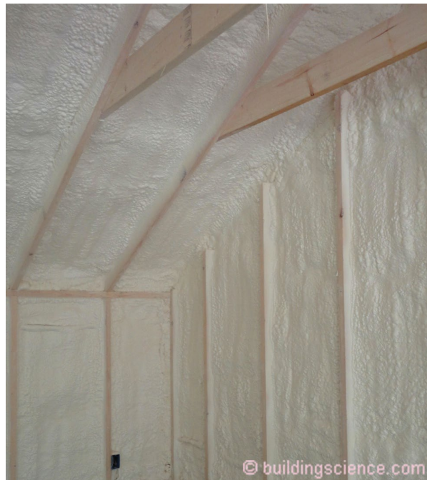
Photograph 1: Closed cell spray foam is often installed on the underside of roof sheathing.
