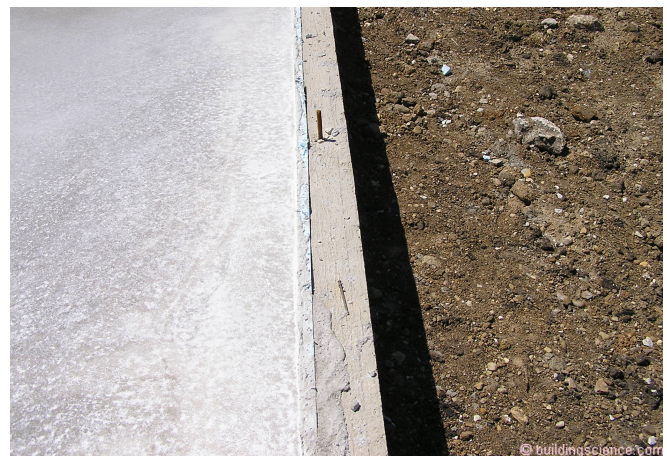
Photograph 3 - Concrete slab is cast. Protective membrane strip yet to be installed. The protective membrane strip should bridge the top of the slab and the top of the stem wall. The protective membrane strip acts as a capillary break providing moisture control and acts as a termite and insect barrier.
