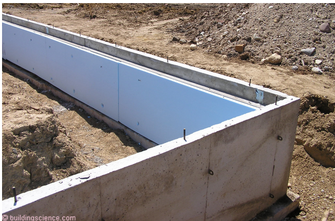
Photograph 1 - Stem wall perimeter foundation insulated on the interior with extruded polystyrene (XPS). Note the depth of the “seat” in the top of the stem wall to accommodate the thickness of the rigid insulation yet to be installed and the thickness of the slab yet to be cast.
