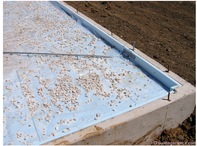
Photograph 2 - Horizontal rigid insulation installed covered with a polyethylene vapor barrier. Note the vertical rigid insulation strip in the “seat” of the stem wall creating a thermal break between the yet to be cast slab and the support for the perimeter exterior wall framing. The stones on the top of the polyethylene sheet are being used to keep the sheet poly from blowing away before the slab is cast.
