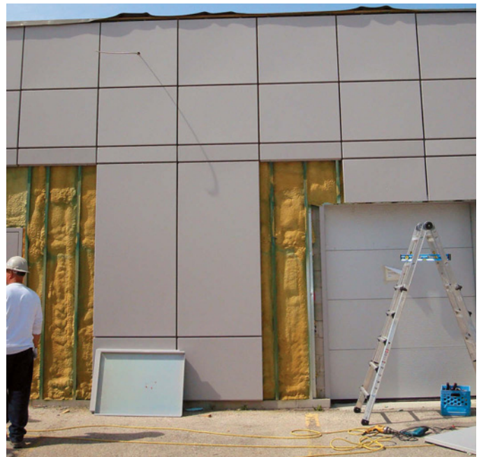
Steel Panel Cladding – Steel panels installed onto wood 2x2 furring embedded in sprayfoam on a masonry wall enclosure for a light industrial strip mall.
