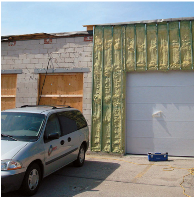
Light Industrial Strip Mall – Masonry wall insulated on the exterior with sprayfoam. Note the treated wood 2x2 furring on screw offsets.
