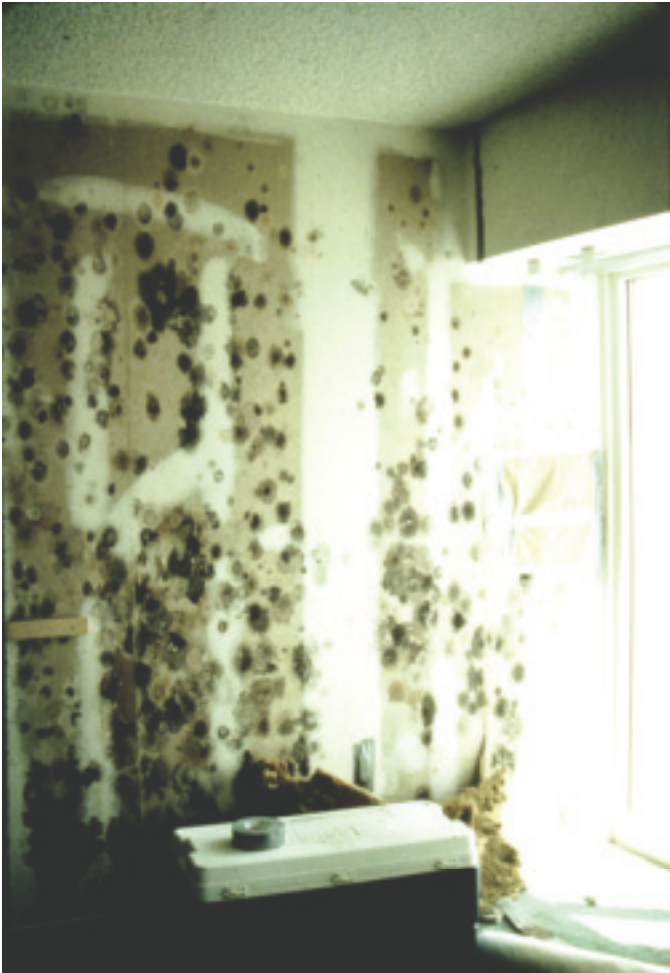
Photograph 6: Demising Wall Mold
