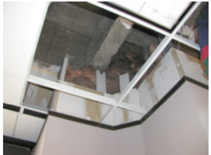
Photograph 2: Lack of Closure
