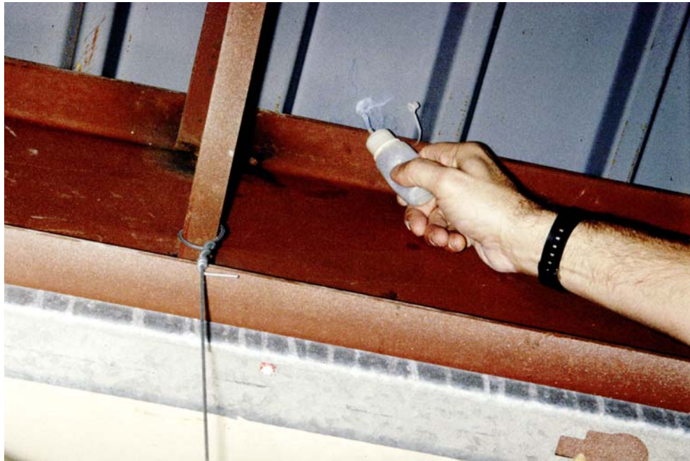
Photograph 3: Negative Pressure In Dropped Ceiling Return Plenum
