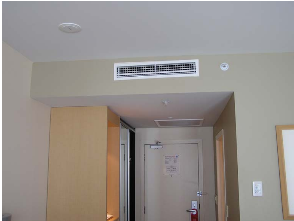
Photograph 5: Fan Coil – Air handler in gypsum board dropped ceiling enclosure
