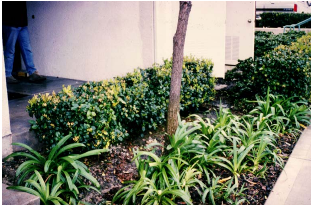
Photograph 6: "Swamp In Desert" Cleverly Located Beside Building Foundation Perimeter
