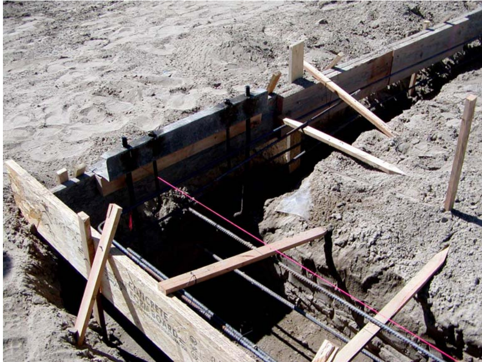
Photograph 8: Sand On Top of Polyethylene – Note polyethylene does not extend to perimeter
