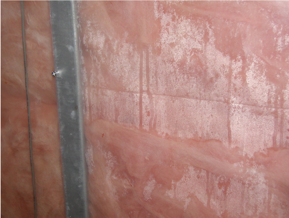
Photograph 1: Interior Polyethylene Vapor Barrier – Condensation from inwardly driven moisture
