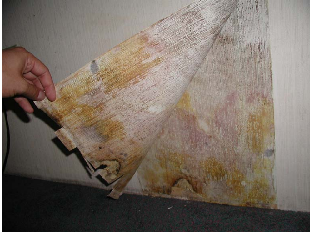
Photograph 2: Vinyl Wallcovering – Mold due to inwardly driven moisture trapped by the vapor impermeability of the vinyl wallcovering
