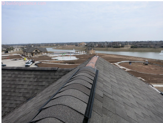
Photograph 2: Vapor Diffusion Port – Non-combustible membrane covering for the vapor diffusion port. The vapor diffusion port materials also need to be vapor open (20 perms or greater – wet cup method and the vapor diffusion port area needs to be 1:150 of the attic area).
