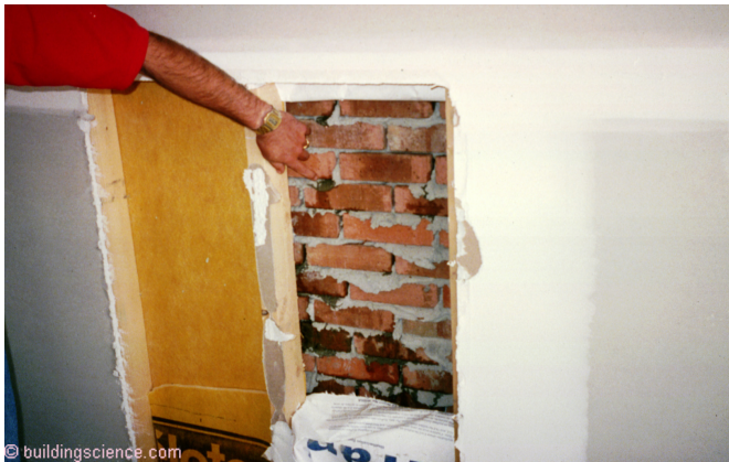
Photograph 2: Water Leakage - In about 20 to 30 seconds water can be seen penetrating and running down the back of the brick. The water penetrates the joints between the brick and the mortar. The water does not pass through the brick or pass through the mortar. The weak link is the connection between the brick and the mortar.
