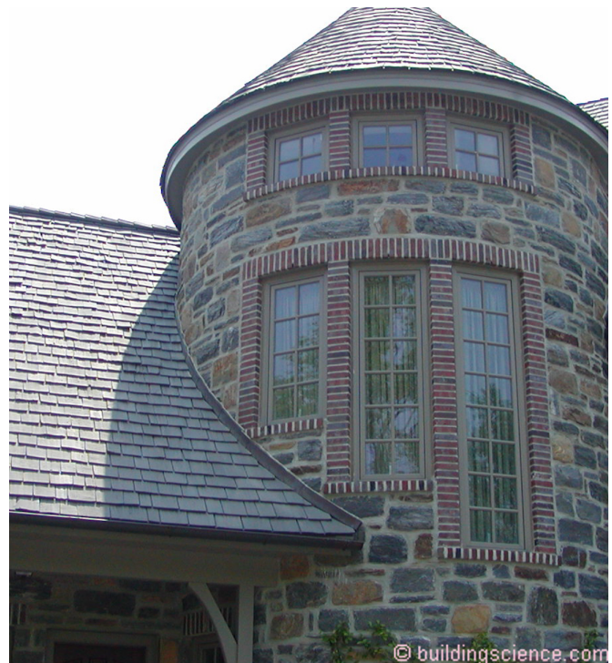
Photograph 12: Stone Veneer - Nothing like a stone turret meeting a roof to have fun with.
