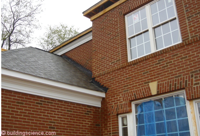
Photograph 9: Walls Meeting Roofs: Where we have the intersection of a sloping roof with a brick veneer wall the water control of the roof needs to connect to the water control of the wall. It is necessary to drain the back of the brick veneer to the exterior. This is not done here. The roof flashing is sealed to the face of the brick.
