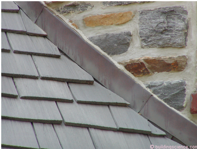
Photograph 13: Sealant Dreams - Yup, a little bit of sealant will do the trick. Hah! The stone has to be removed and through wall flashing installed.
