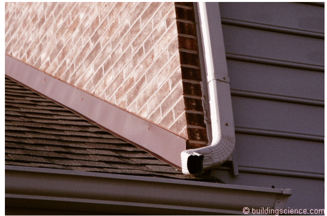
Photograph 11: Counter Flashing Does Not Work – For the counter flashing to work it has to be connected to a through wall flashing that then connects to the water control layer of the wall.
