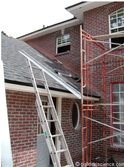
Photograph 10: Regletting Does Not Work - Saw cutting a “notch” or “reglet” into the brick and inserting a “counter flashing” will not do the trick. No chance.
