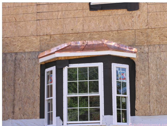
Photograph 5: Bump Out Approach One - Copper roof with an integral roof is installed first, before the brick veneer and before the water control layer. Easy, elegant and it works. So why not this approach all the time? Ah, it is a pain in the butt to protect the metal roof while the brick is installed. It tends to get damaged...and so the builders want to install it after the brick.
