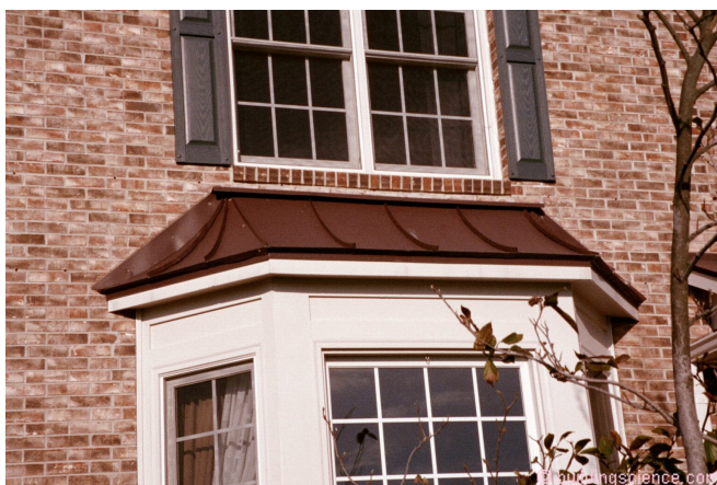
Photograph 4: More Bay Bump Outs - Same thing is going on here. The roof flashing is sealed to the face of the brick. It does not penetrate through the brick and connect to the water control layer behind the brick.
