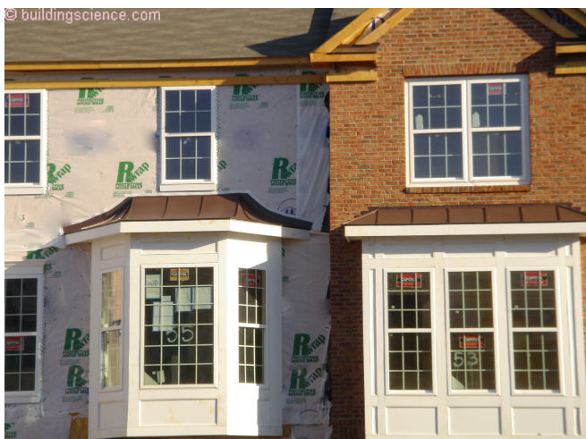
Photograph 3: Bay Bump Outs - Two bay bump outs are shown. The vinyl siding has not yet been installed above one bay bump out, but the brick has been installed above the other. The metal roof flashing is sealed to the plastic membrane water control layer in the wall where the vinyl siding is to be installed. In the brick wall, the metal roof flashing is sealed to the face of the brick veneer. The flashing does not penetrate through the brick and connect to the plastic membrane water control layer behind the brick.
