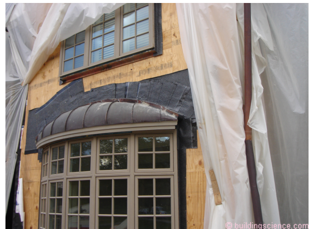
Photograph 8: Stone Veneer Bump Out Repair - The stone had to be taken down and a membrane installed to connect the water control of the metal roof to the water control of the wall.
