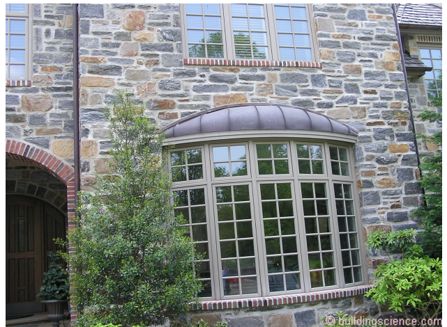
Photograph 7: Stone Veneer Bump Out - Metal roof sealed to the face of a stone veneer. Bad, bad, bad....
