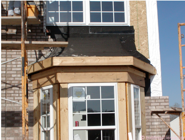
Photograph 6: Bump Out Approach Two - A fully adhered water control layer is installed prior to the installation of the brick and prior to the installation of the metal roof over the bay. This type of membrane is typically “robust” enough to survive the installation of the brick veneer. When the metal roof is installed over the top of this water control layer membrane, after the brick veneer is installed, it does not need to pass through the brick.
