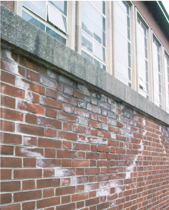
Photograph 4: Getting It Wrong Turning into Ugly— Efflorescence and freeze-thaw damage occurring and the cause is a combination of bad water control and bad brick. Could good brick have survived the bad water control? Maybe. But with good water control even the bad brick would have lived.
