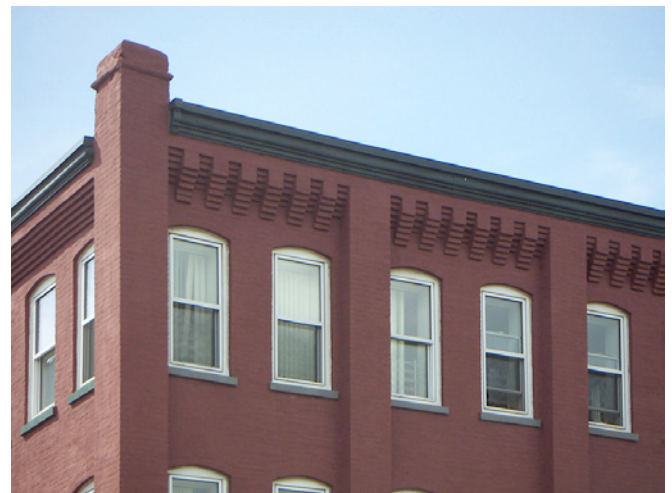
Photograph 9: Back Side Brick —Brick on the back side was stuccoed with a polymer cement slurry. The thin vapor open hydrophobic cementitious layer allows the texture of the brick joints to show through. It is real important that the vapor transmission of the cementitious layer is greater than 10 perms. If not the coating will bubble and blister and peel. An even more conservative approach is the European one—just add a direct-applied traditional stucco and forgo the historic tax credit.
