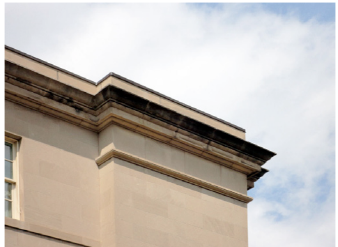
Photograph 7: Courthouse in Washington— Can't tell you which one or I will end up in jail. And not just any courthouse—an unbelievably beautiful courthouse—but a parapet without a drip edge. Look at the stains. Criminal. The fix is in Figure 3.
