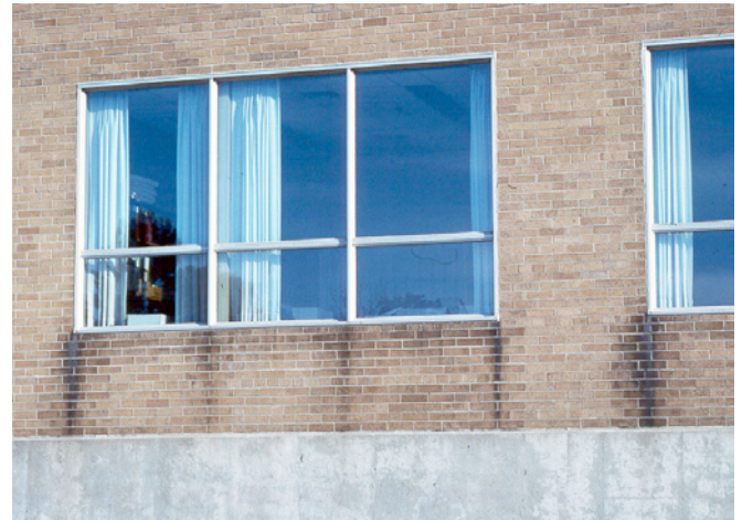
Photograph 2: Getting It Wrong —Look at the stains. Large expanses of glass don’t absorb water and water runs down them and ends up at corners that are typically “inset” with surfaces that don’t slope. It gets worse, the windows themselves leak. Look at the bottom of the mullions where they meet the sill.
