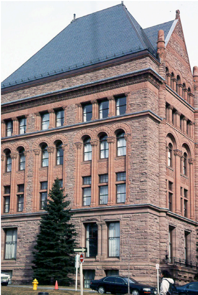
Photograph 1: Getting It Right —Classic building at University of Toronto “Romanesque”. Look at all the drip edges – at roof edges, at window openings, between floors. Notice that they are working. How can you tell? No stains. Look at this building carefully because it is an example of “what is good”.
