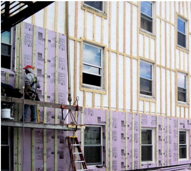
Photograph 8: Next Step — Add the rigid insulation. Layer it between the furring and then over the entire kit and caboodle in continuous layers.
