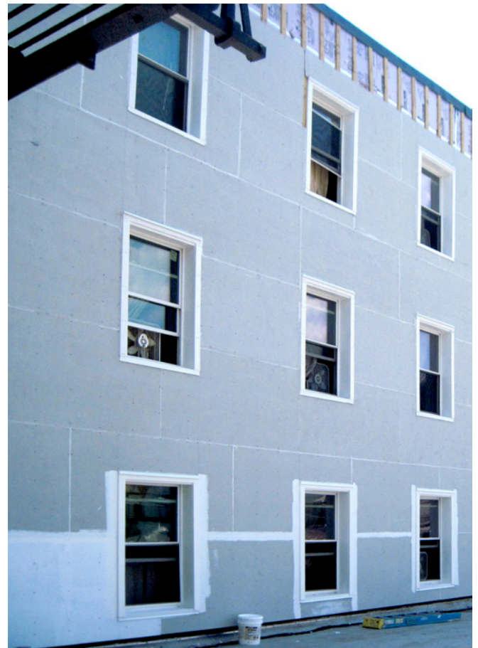
Photograph 10: More Fiber cement Panels —Note the “innie” windows. I don’t always win.
