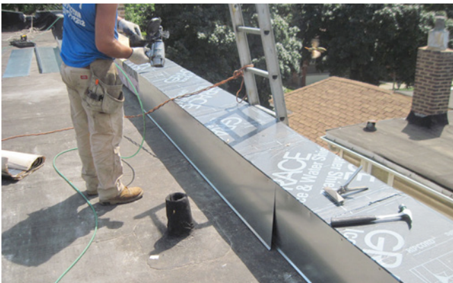
Photograph 6: Parapet Water Proofing —Don’t forget the drip edges. And don’t forget the counter flashing.
