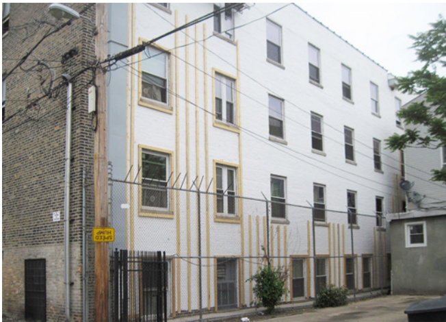
Photograph 7: Jumbo Sequencing —With the jumbo sized buildings you just start on one side and work your way around. First the fluid applied water control layer and air control layer and the 2x4 wood furring.
