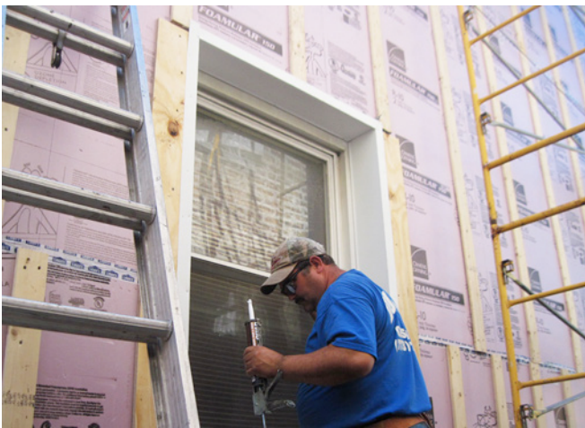
Photograph 12: “Innie” Window —The best argument for “innies” is that the existing windows are good enough not to be replaced as part of the retrofit. If you are replacing the existing windows with new high performance windows the best option is an “outie.”
