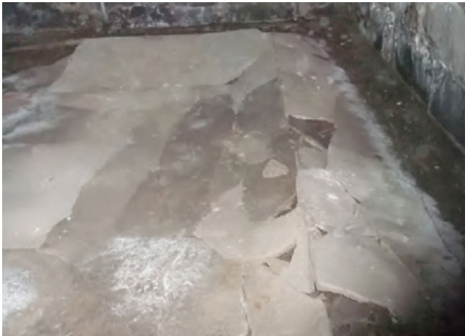
Photograph 1: Slab Heaving in Unheated Basement —So why didn't the walls collapse inwards and only the slab buckled upward? Easy, the ground beside the foundation wall was not wet, only the ground under the slab was wet. Another "ah ha" moment. You need wet soil for frost heave. Not only do you need wet soil, you actually need "frost-susceptible" wet soil. A miserable type of soil with an annoying distribution of fines. The size of voids in a soil determines its frost-susceptibility. More than 3% grains finer than 0.02 mm in diameter by weight usually are a problem.
