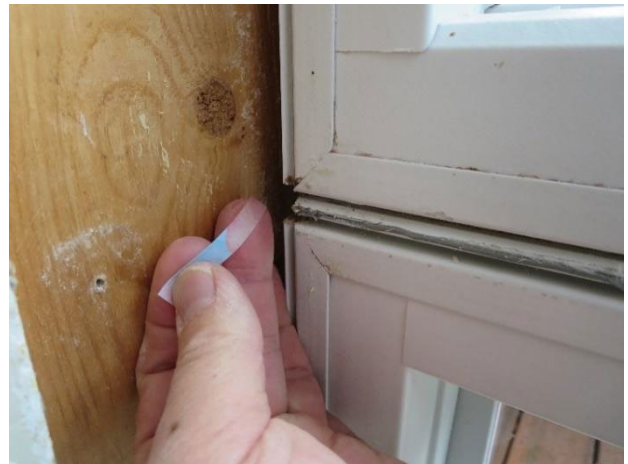
Figure 50: Water leakage due to injection
