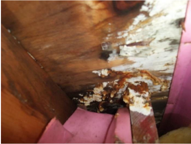
Figure 22: Poorly vented cathedral roof fungus
