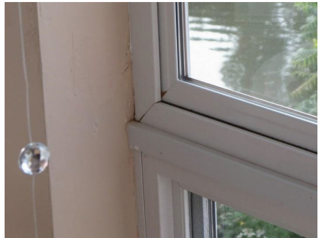
Figure 42: Damage at jamb at mull joint
