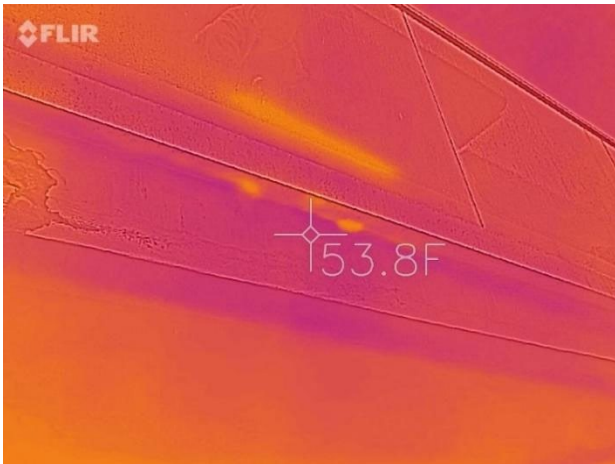
Figure 57: Visual and infrared image of incorrectly-draining glass railing detail (no drainage gap)
