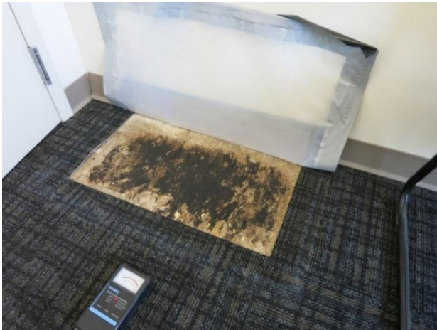
Figure 26: Subfloor discoloration under carpet tile at slab-on grade condition
