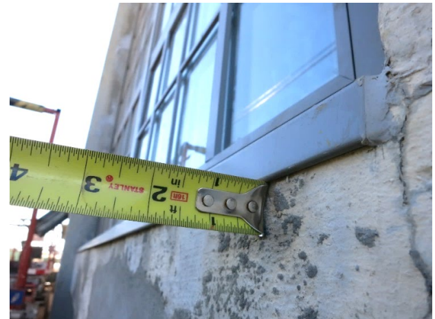
Figure 15: Sill drip edge pushed against wall
