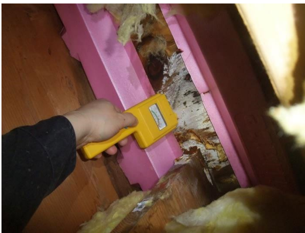
Figure 23: Delmhorst meter at roof sheathing
