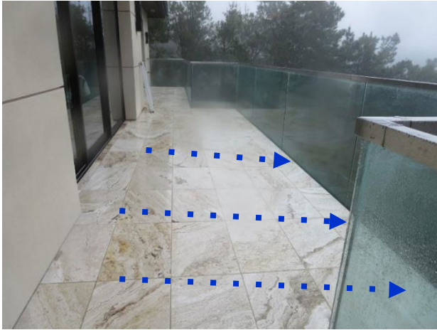
Figure 54: Water drains off face of balcony
