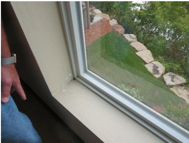
Figure 40: Damage at bottom window corners
