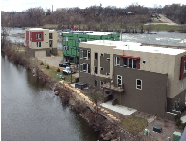
Figure 39: Residences with window leak issues
