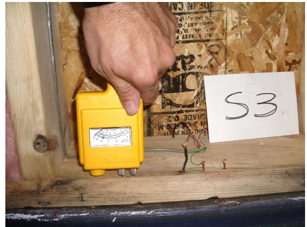
Figure 21: Delmhorst meter at interior of sill plate
