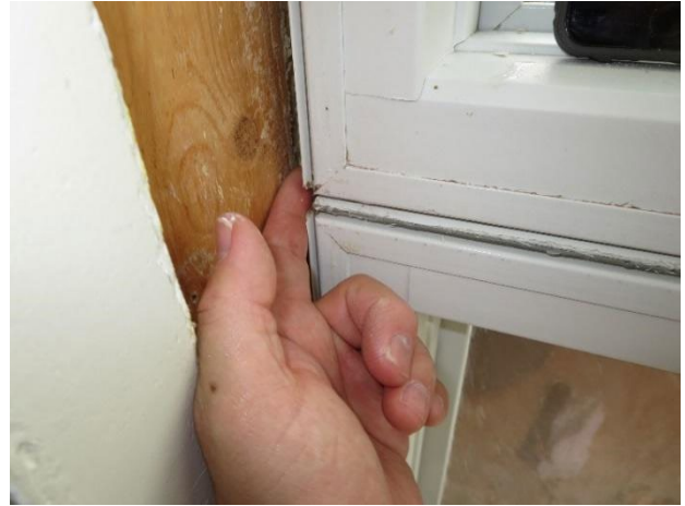
Figure 45: Water leakage coming in at mull joint
