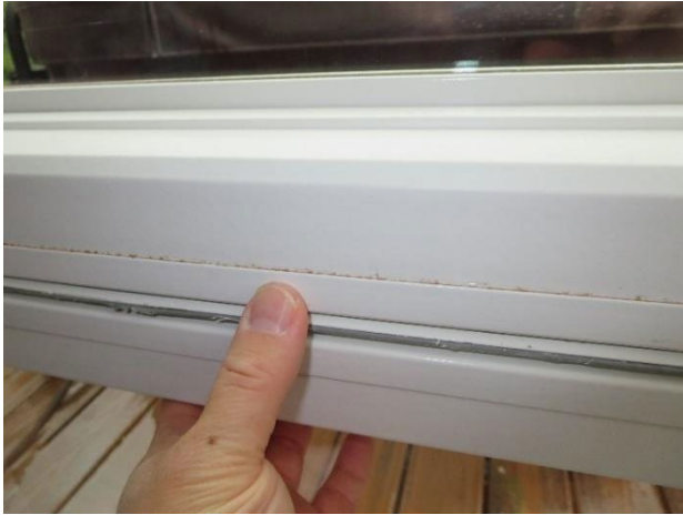
Figure 47: Water pushing on vinyl joint
