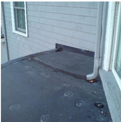
Figure 51: Water leakage at roof/ceiling insulated with open cell spray foam; EPDM roof-to-wall joint
