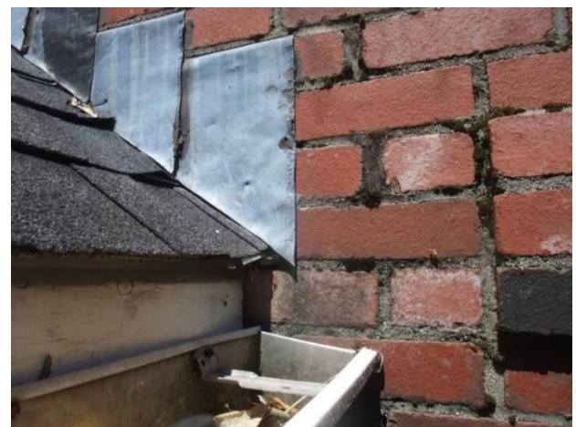
Figure 3: Moss growing on brick mortar joints
