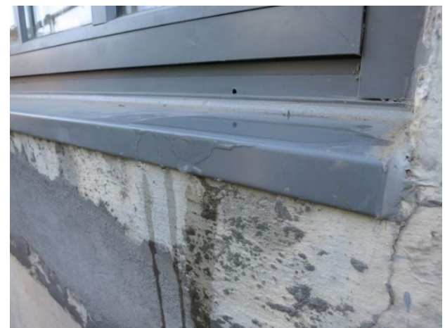
Figure 16: Window runoff spills onto wall below
