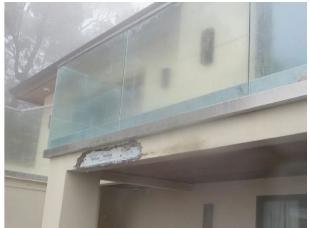
Figure 53: Leakage into stucco soffit below
