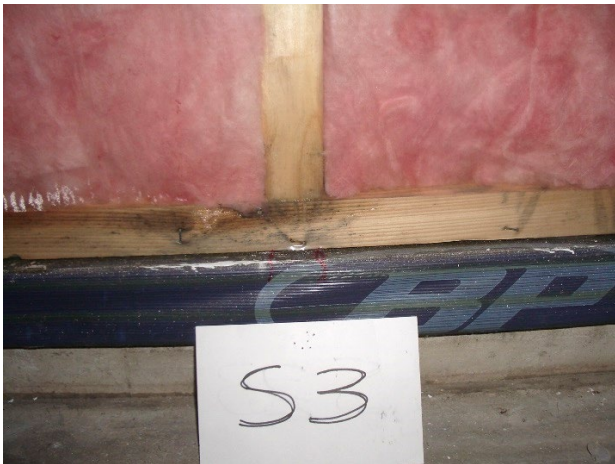
Figure 20: Test hut sill plate soaked with water
