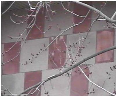
Moisture damage to signature masonry cladding
