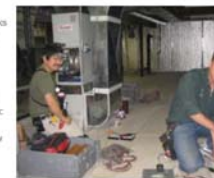
Image 1 of 9 A tankless water heater provides space heat for the whole house. Two energy specialists from the Building Science Corporation, Kohta Ueno and Armin Ruedl, install an air handler equipped with a hydronic heat exchange coil in one of the homes enrolled in a deep-energy-retrofit project in Utica, New York.
