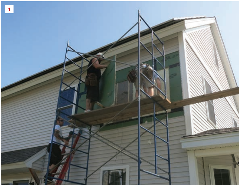
1. After three seasons of moisture and temperature monitoring, workers pull sections of Zip sheathing panels from the test wall section of a house in Devens, Mass.
