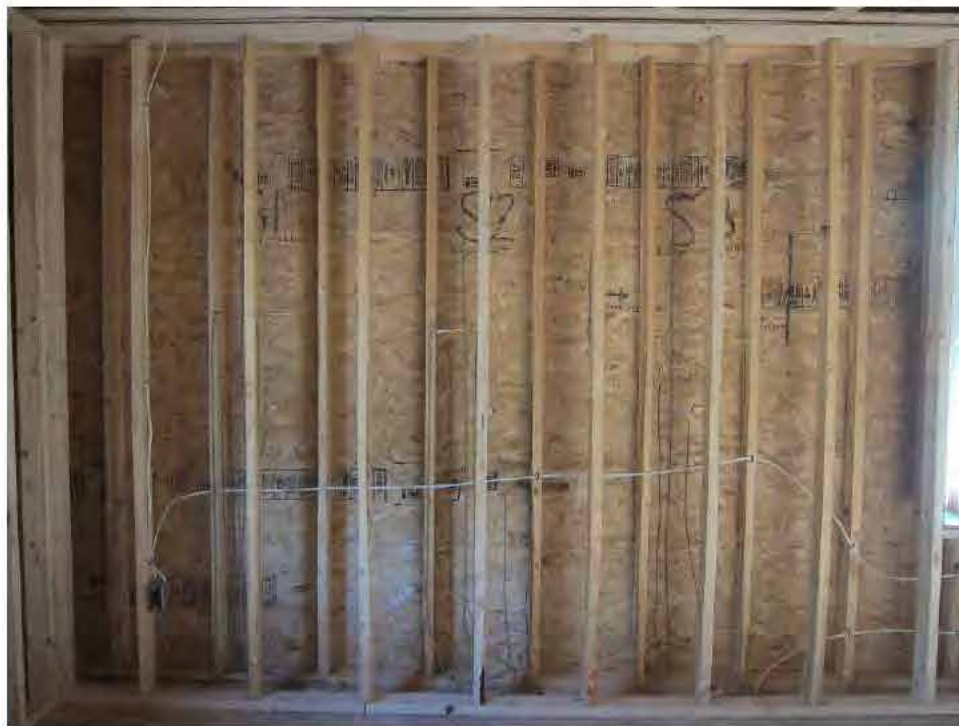
Figure 50. South test walls after installation of sensors, showing double-stud layout The test wall instrumentation plan for this research is shown in Figure 51.
