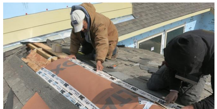
Photograph 2: Vapor Open Layer – Port opening in the roof deck covered with a water tight and airtight but vapor open layer.
