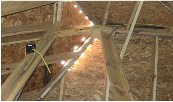
Photograph 5: Round Port Openings at Hip Roof – View from underneath the roof assembly showing the location of the round port openings at the upper part of the hip roof assembly.
