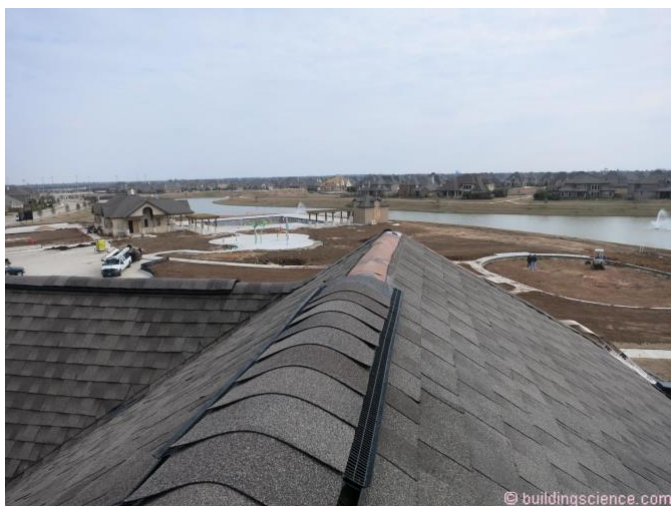
Photograph 3: Standard Ridge Vent – A standard ridge vent is installed over the water tight and airtight and vapor open layer.
