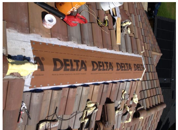
Photograph 4: Tile Roof Opening – Watertight and airtight and vapor open layer being installed.
