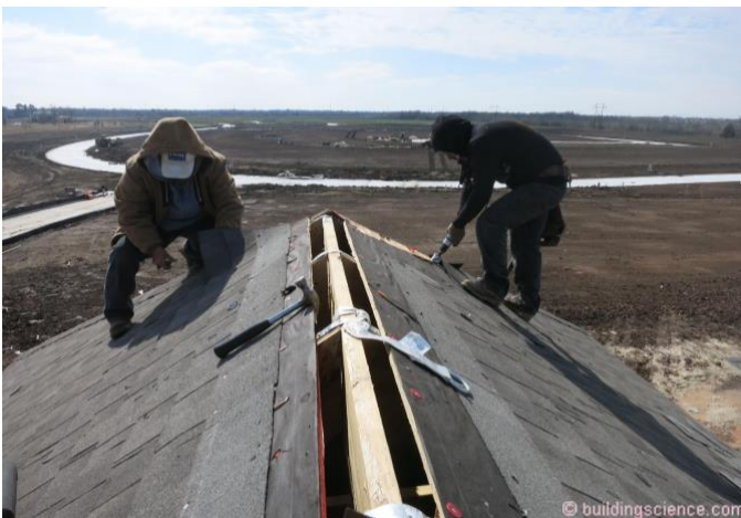
Photograph 1: Vapor Diffusion Port (Strip Port Openings) Asphalt Roofs - Standard roof vent opening located at the ridge.
