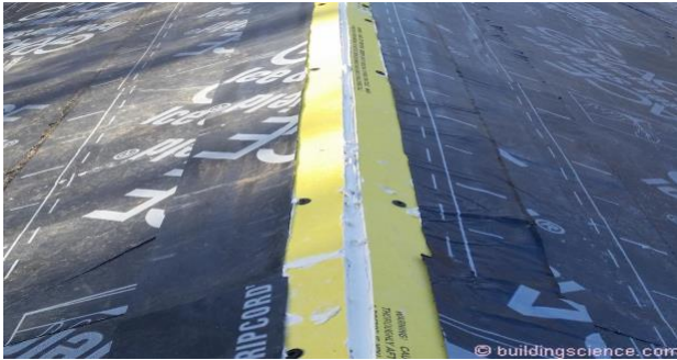
Photograph 6: Fireproof Diffusion Port Layer – Exterior rated gypsum board can be used for the water tight, air tight and vapor open layer.
